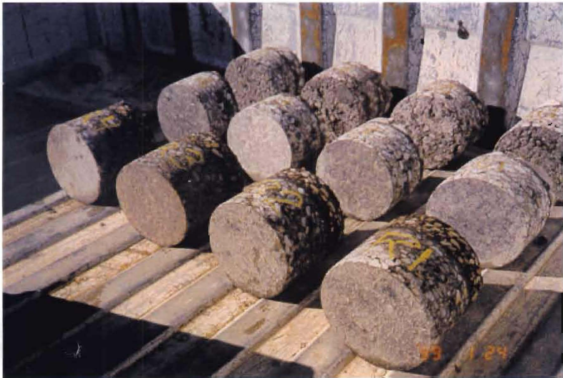
Photos showing the difference in surface texture six months after treatment (untreated – back; CRF – middle; Reclamite – front)
