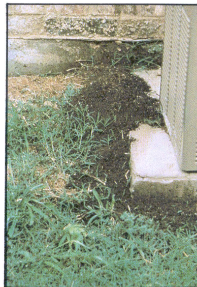
Fig. 24, above. Fire ants are attracted to electrical equipment for unknown reasons. They are a major problem for heat pumps, transformer boxes and air conditioners where they can short out electrical circuits. They can sometimes chew through electrical cable insulation, causing shorts in telephone lines and traffic lights.
