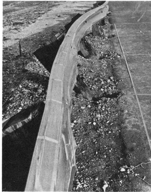
Figure 1. Typical guardrail installation after vehicle impact.
