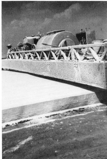
FIGURE 35. EQUIPMENT USED TO APPLY CURING COMPOUND TO FRESHLY LAID CONCRETE PAVEMENT; COMPOUND HAS BEEN APPLIED TO CONCRETE IN LEFT FOREGROUND.
