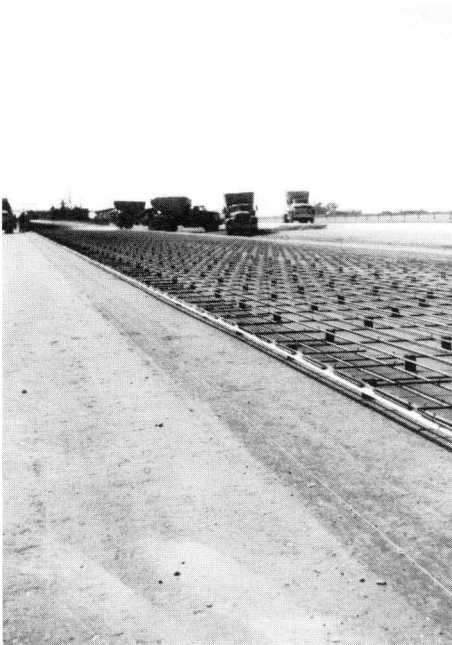
FIGURE 27. WET BATCH TRUCKS DELIVERING CONCRETE TO JOBSITE. SURFACE OF ASPHALTIC CONCRETE LEVEL-UP IS BEING WET DOWN IN LEFT REAR, AHEAD OF PAVING TRAIN.
