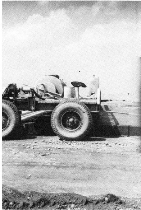
FIGURE 34. SIDE VIEW OF EQUIPMENT USED FOR APPLICATION OF CURING COMPOUND TO SURFACE OF WET PLACED CONCRETE.
