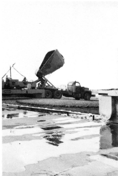
FIGURE 29. CONCRETE BEING DELIVERED TO #2 SPREADER; BACK END OF #1 SPREADER IS AT RIGHT. HOT-MIX ASPHALTIC CONCRETE LEVEL-UP CAN BE SEEN IN FOREGROUND.
