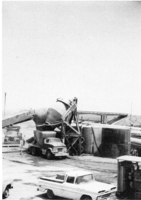
FIGURE 24. TWO 9-YARD MIXERS OF 540 CU YD HOURLY CAPACITY AT CENTRAL MIX PLANT. ALL BATCH INGREDIENTS ARE FED TO MIXERS BY CONVEYOR AT LEFT.
