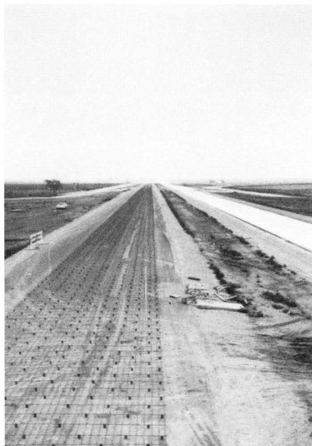
FIGURE 55. LONG STRETCH OF CONTINUOUS REINFORCING STEEL MAT FABRICATED FROM DEFORMED STEEL BARS. PAVEMENT WIDTH IS 24 FEET; BASE COURSE IS HOT-MIX ASPHALTIC CONCRETE.
