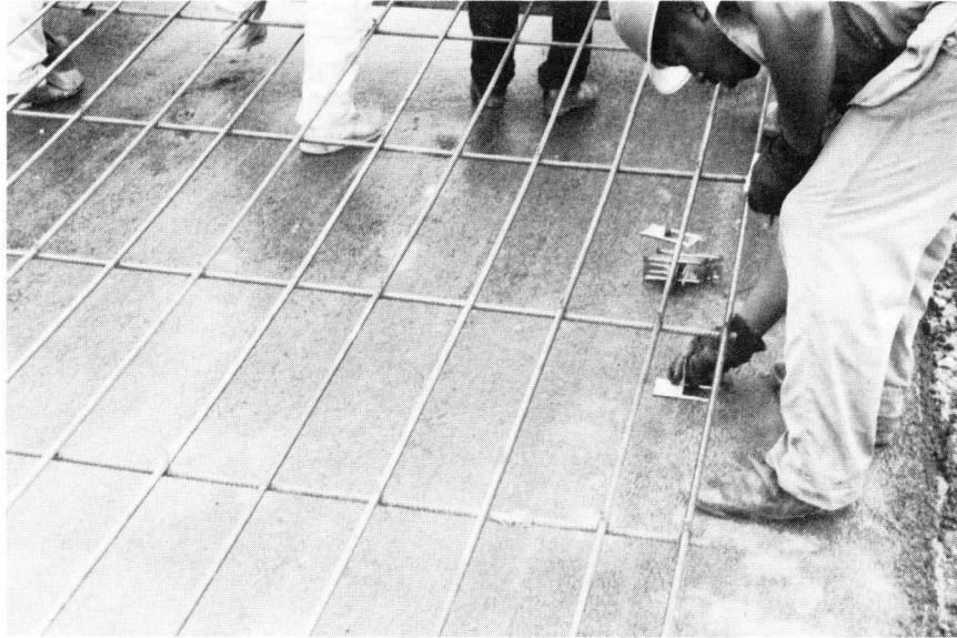
FIGURE 50. PLACING SHEET STEEL CHAIR FOR EDGE SUPPORT OF TIED DEFORMED STEEL BAR MAT.
