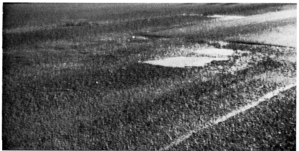
Figure 1—Eroded spot in a hot-mix asphaltic overlay on a portland cement concrete base after eighteen months' service.
