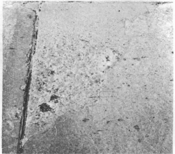
No. 8 after six months service. Surface wear is evident in wheel path.
