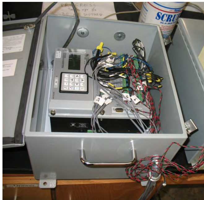
Figure 6-7: Steel box for data logger
