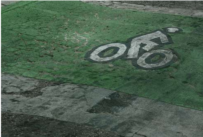
Figure 19. Poor quality of road led to the deterioration of the thermoplastic bike boxes on Speedway
