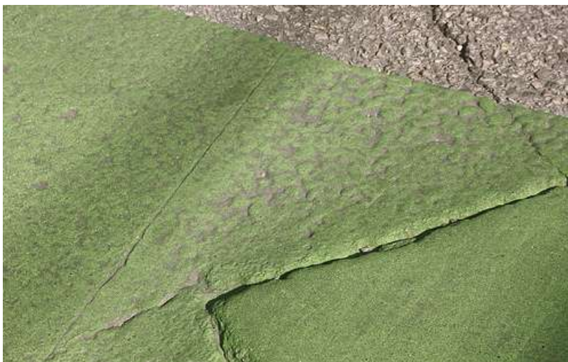
Figure 20. Thermoplastic thinning on the colored lane on San Jacinto Boulevard
