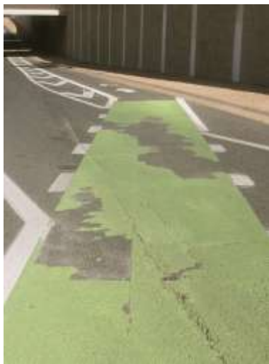
Figure 18. Deteriorating thermoplastic on Dean Keaton Street at one of the I-35 exit ramps (breaking up in sheets)
