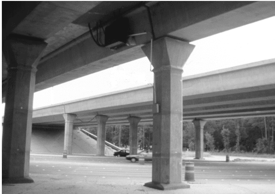
Figure 3.19 - DAS Box with Companion Access Box (Louetta)
