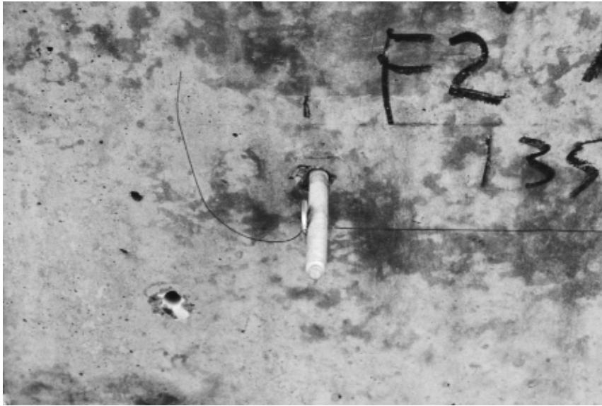
Figure 3.7 - Dead (Anchorage) End of Tensioned-Wire Deflection System
