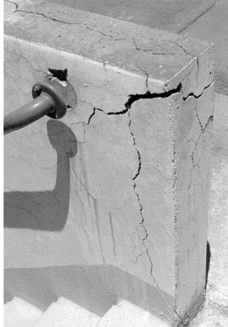
Figure 2.13: Severe Concrete Cracking Attributed to Delayed Ettringite Formation
