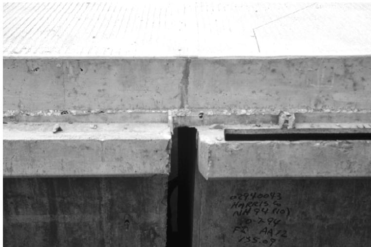
Figure 11.17: Blow-Up Detail of Deck Cracking between U-Beams at Interior Bent Support
