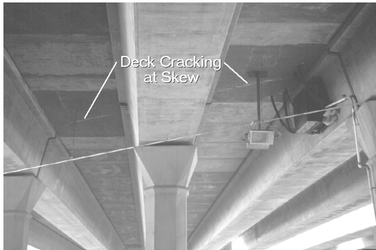
Figure 11.18: Deck Cracking at Skew between Mainspan U-Beams
