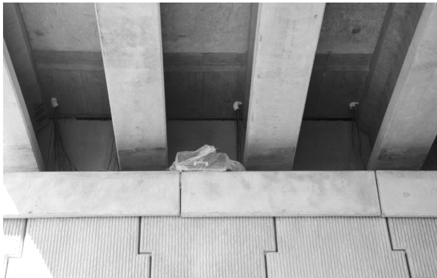
Figure 9.5: Location of Data Acquisition System at Bridge Abutment
