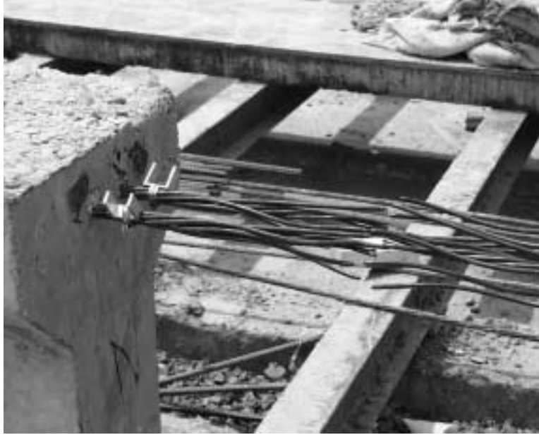
Figure 9.4 Flame Cut Strands and Unwinding of Ends
