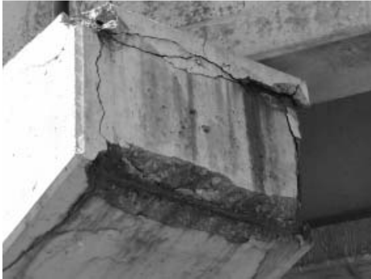
Figure 5.8 Damage to an endcap of Structure #5
