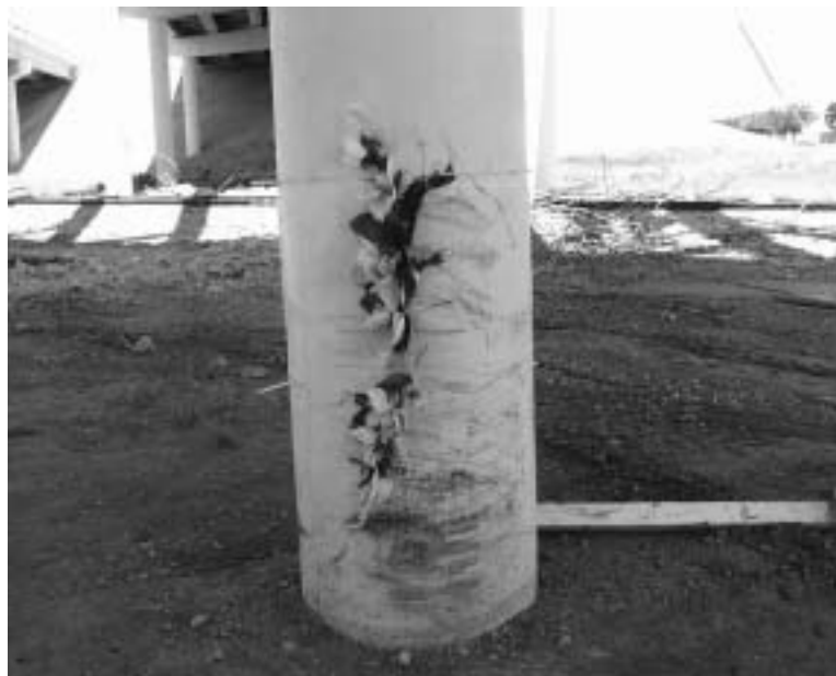
Figure 7.7 Vehicular collision damage on column of Structure #2
