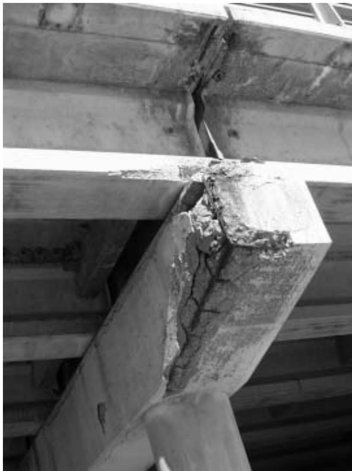
Figure 5.9 Delamination on an endcap of Structure #8
