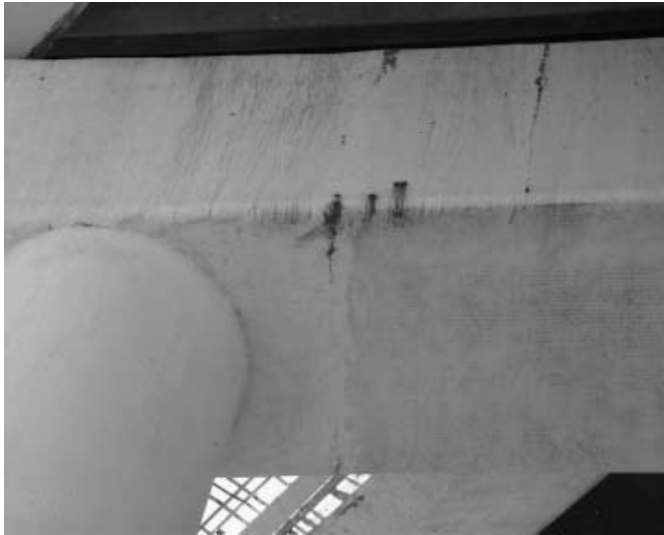
Figure 7.8 Rust stains on bent of Structure #1
