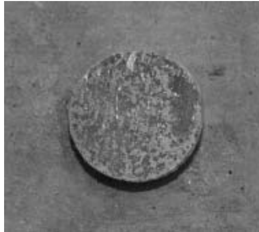
Figure 6.12 Failure at the epoxy/concrete interface on Test #2
