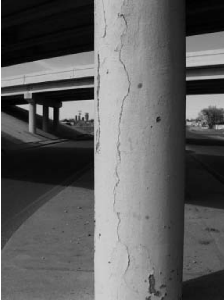
Figure 5.10 Cracking on column of Structure #12
