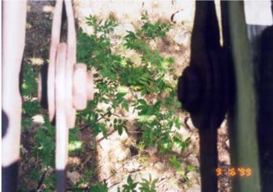
Figure A.11: Bottom chord joint L1
