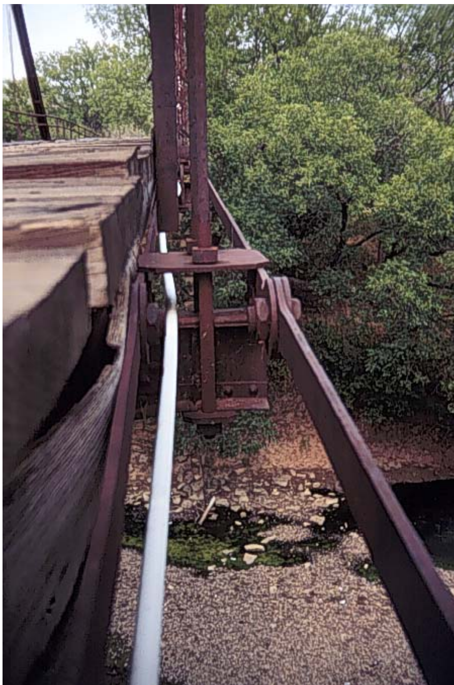
Figure A.9: Bottom chord joint L1
