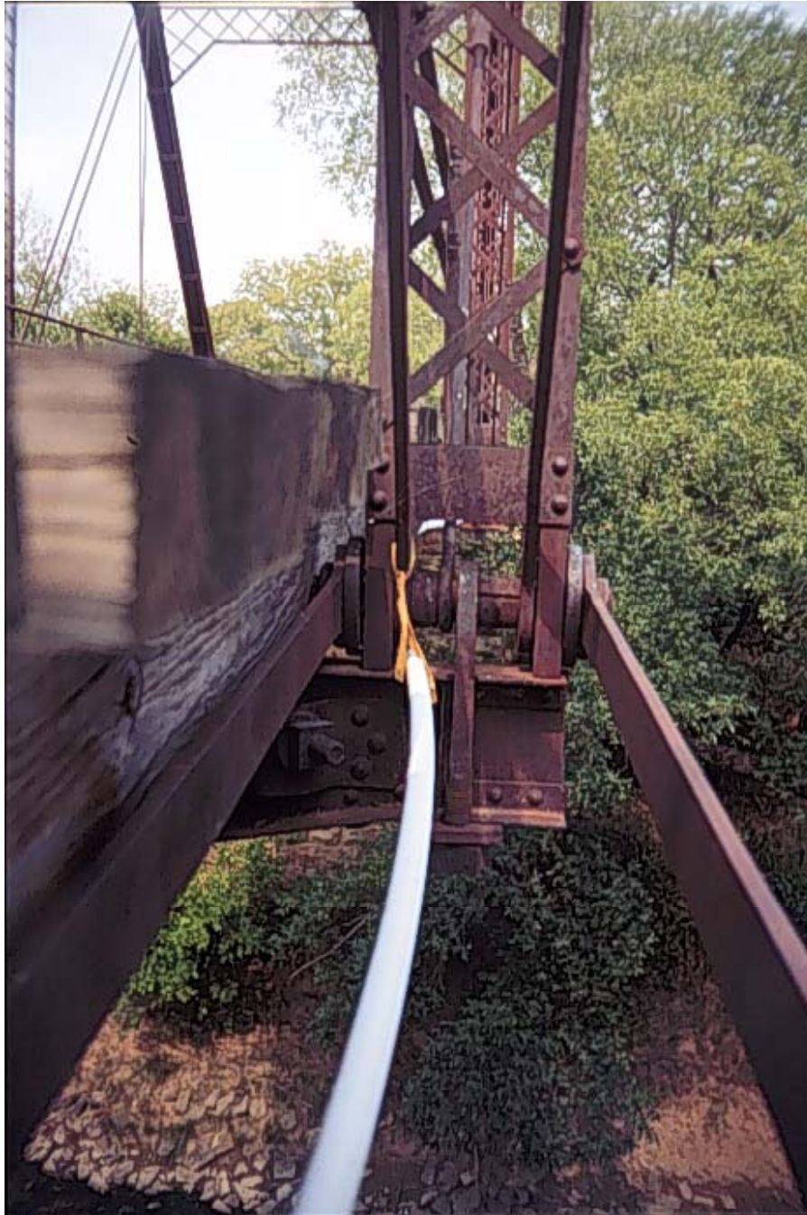
Figure A.10: Bottom chord joint L2
