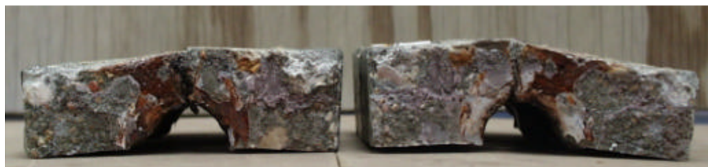
Figure 4.24 Incompletely Filled Epoxy Joint (SE-S-M-CI-1).
