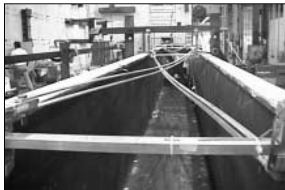
Figure 4.14 Bracing Slack during Initial Loading
