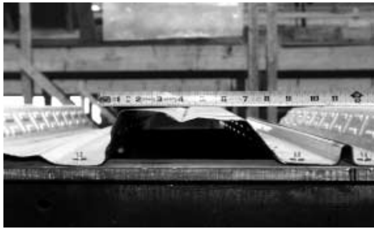
Figure 8.2 Metal Deck Distortion
