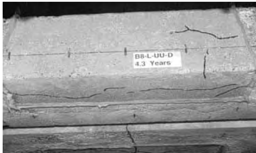
Figure 2.32 Cracking on non-precracked beam B8.
