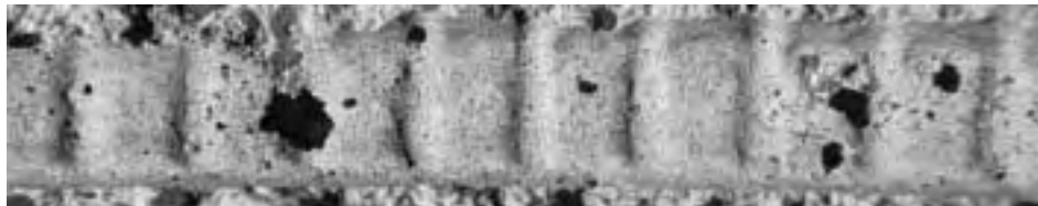
Figure 2.89 Stirrup trace in concrete.
