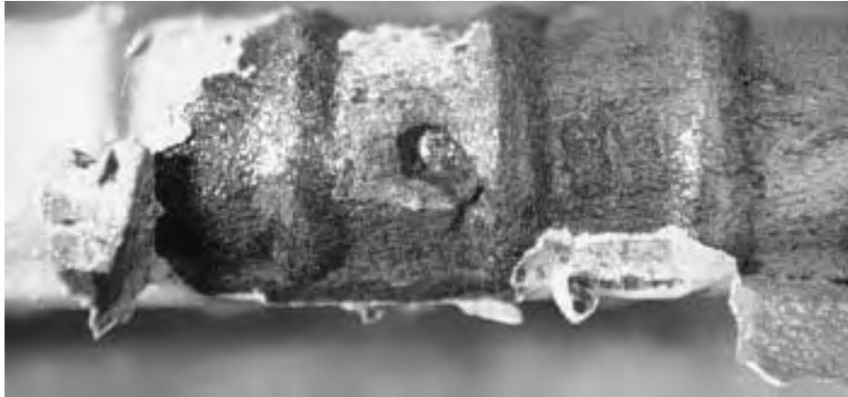
(a) Pitting on upper longitudinal bar
