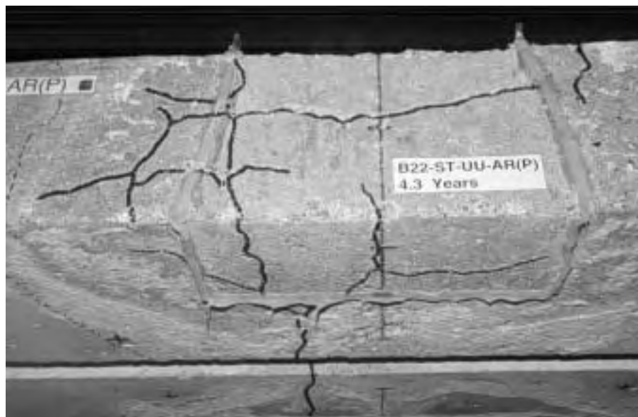
Figure 2.36 Random cracking on non-precracked beam B22.
