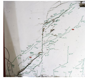
(b) Crack patterns of IV-1.2-03-V
