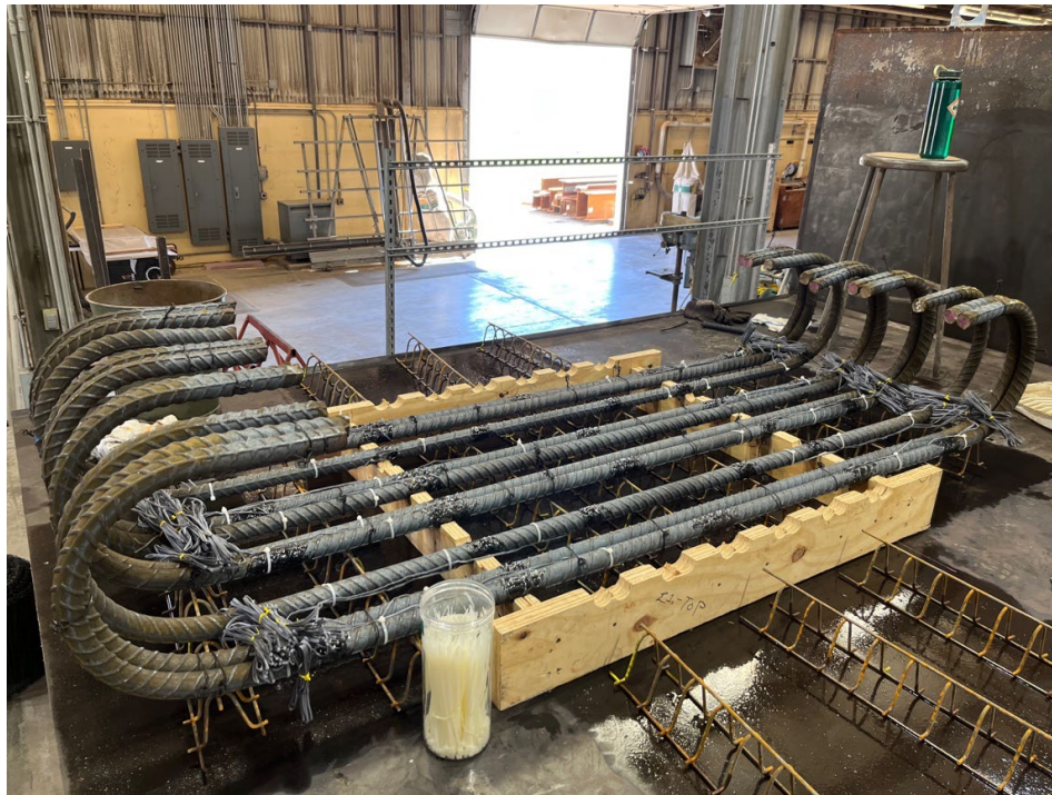
Figure 6-8 First phase bottom mat reinforcement fabricated on top of the bottom segment of wooden formworks
