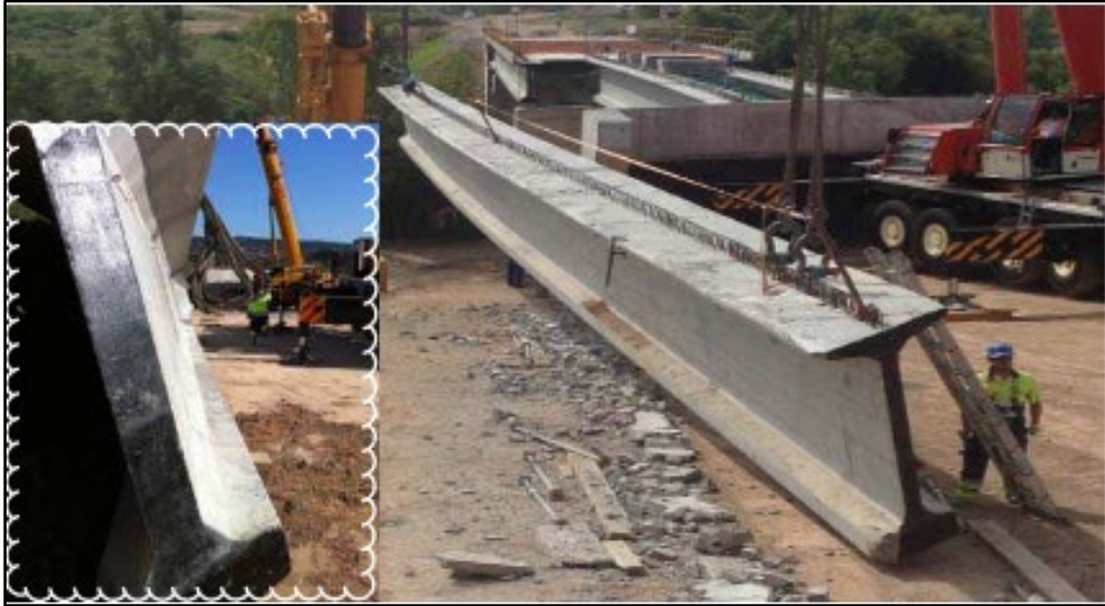
Figure 2.14. Lifting Failure, Fuente et al. (2018)
