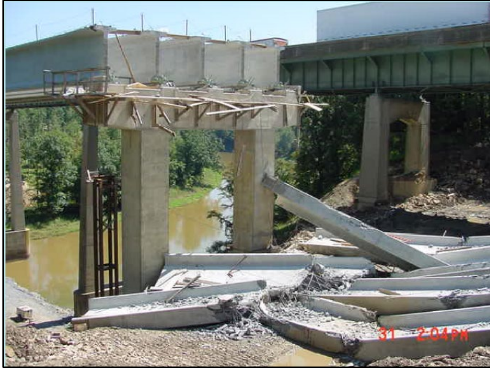
Figure 2.16. Failure of erected girders, courtesy of TxDOT
