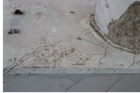
(b) Torsional cracks
