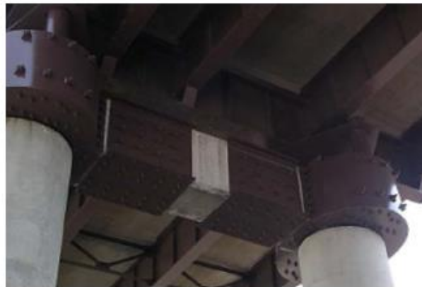
Figure 2-23. Steel jacketing application on a bent cap in Missouri (Wright et al. (2011))
