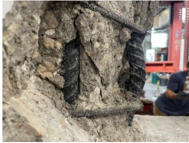
(a) Column long. bar buckling (S-NS-CIP-NH*)
