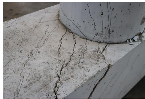
(b) Torsional cracks and crushed concrete
