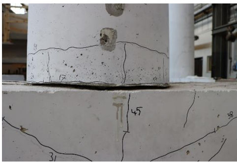
(a) Interface crack
