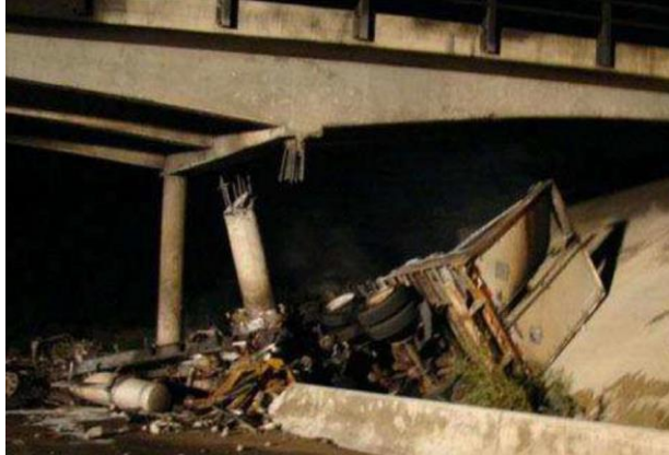
Figure 2-2. Failure of a pier located in bent cap connection caused by truck impact in Colorado (Gallegos and McPhee, 2007)
