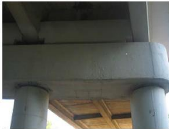
Figure 2-22. Concrete encasement of a bent cap in Tennessee (Wright et al. (2011))
