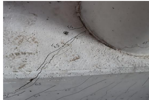
(b) Torsional cracks
