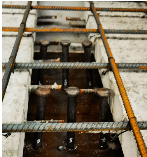
Figure 5.8 - Shear Studs Bent Inward in Specimen No. 2
