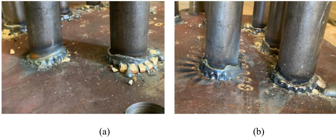
Figure 4.37 - 1-1/8" Studs Welded Without Surface Preparation and Without Cable Looping. (a) lift is 1/8" (b) Lift is 3/16".
