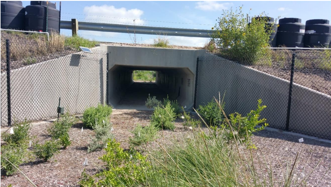
Figure 4.5. Native plants in front of wildlife crossing on SH 100 in Pharr District. Photo courtesy of L. Loftus-Otway
