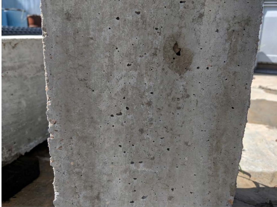
(a) Cracking Index - 0.01 in/yd (Visual Rating – 1.5)
