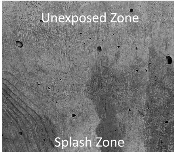
CI-0.015 in/yd, VRI- 1.5) (b) Cracking in area between Unexposed and Splash Zones
