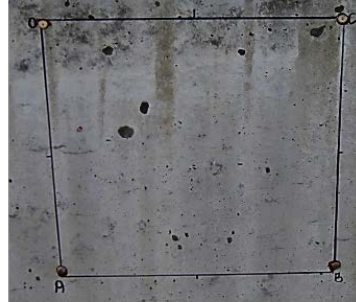
Cracking Index - 0.003 in/yd
