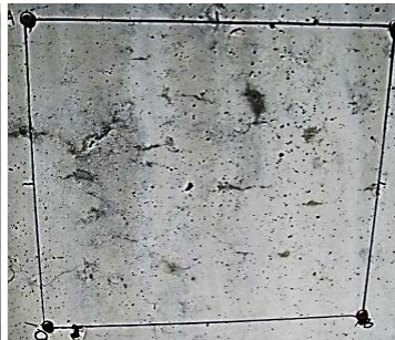
Cracking Index - 0.025 in/yd
