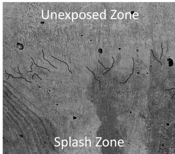
(c) Highlighted Microcracks
