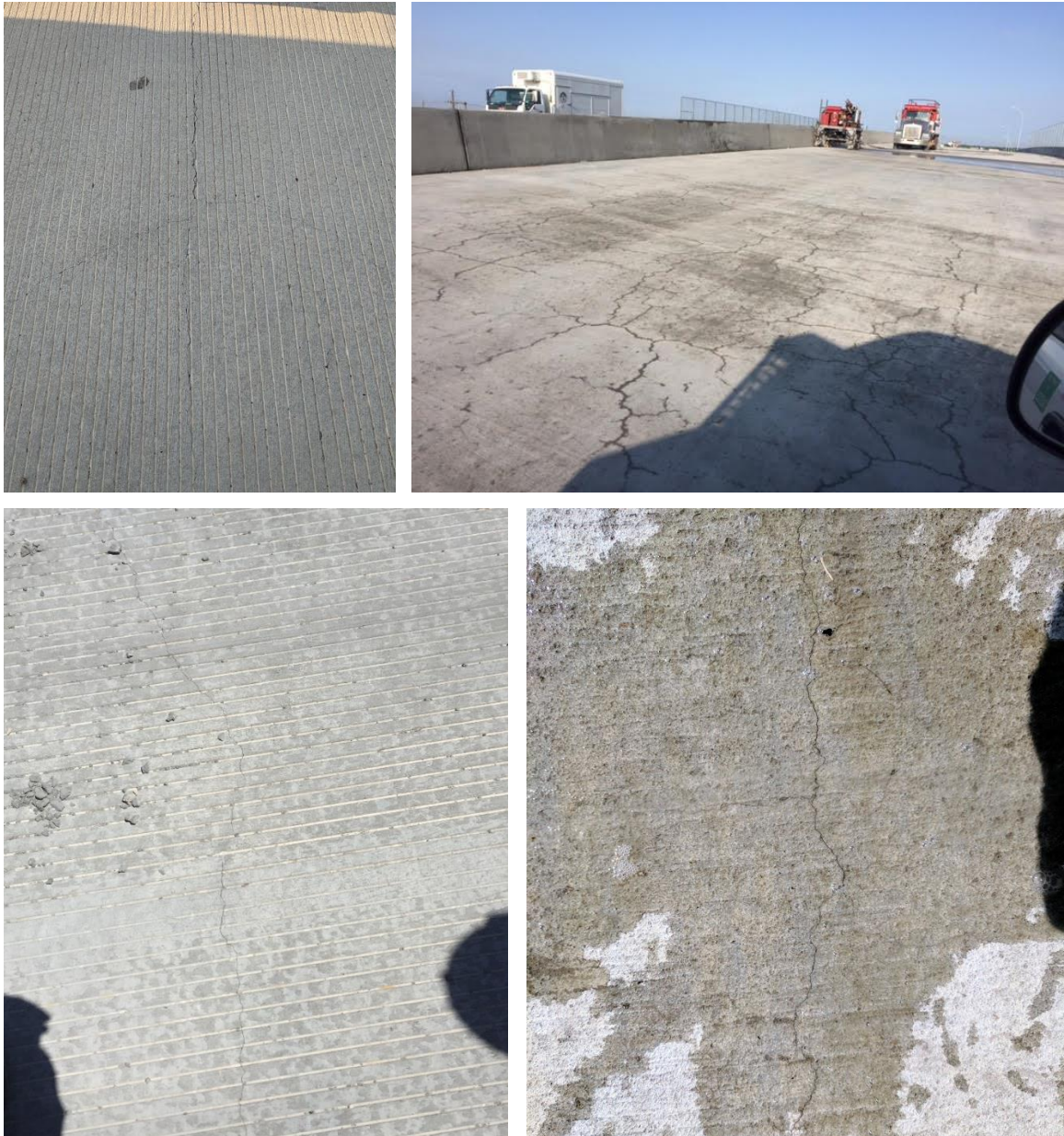
Figure 7.8 Typical cracks observed on Loop 335 bridge deck
