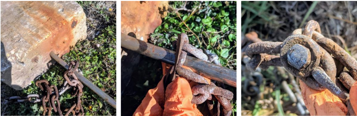
Figure 3.3 Galvanic corrosion (left), loss of cross section (middle), and chain/bolt abrasion (right)
