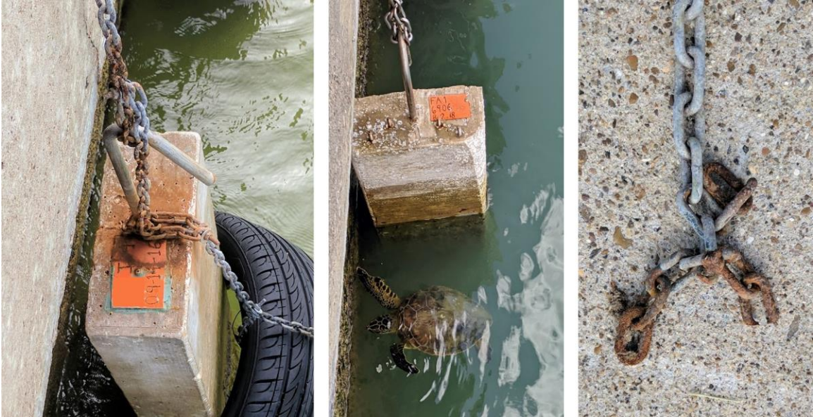
Figure 3.2 Galvanized chain corroding & rubber tire (left), visible abrasion on block corners (middle), and galvanized chain failing (right)
