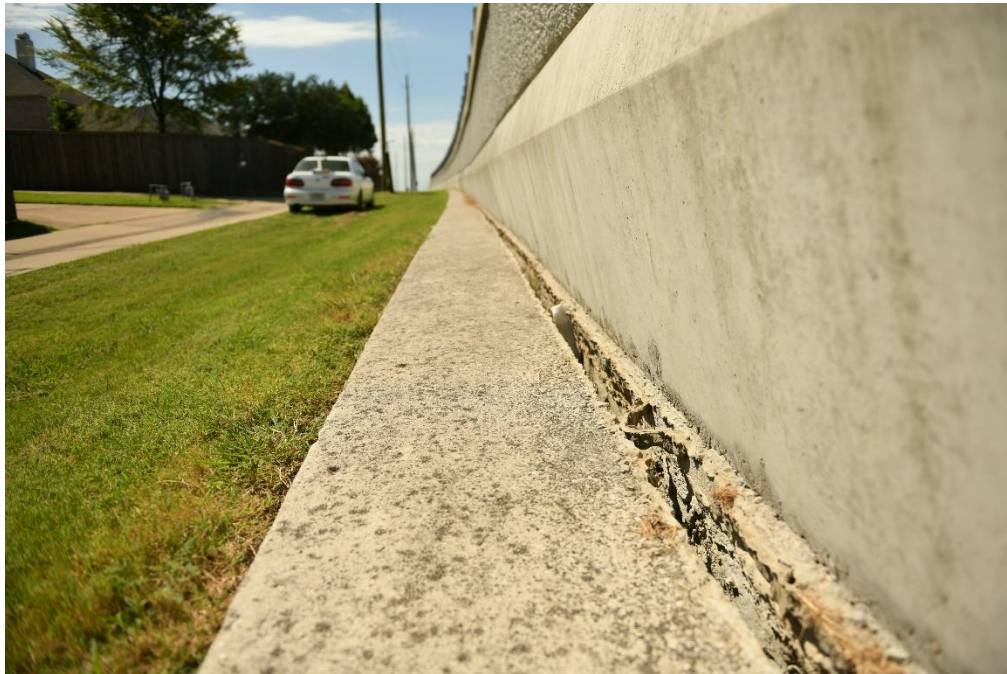
Figure 7.37 Separation between noise wall and concrete base, east side wall, close to receiver R#1
