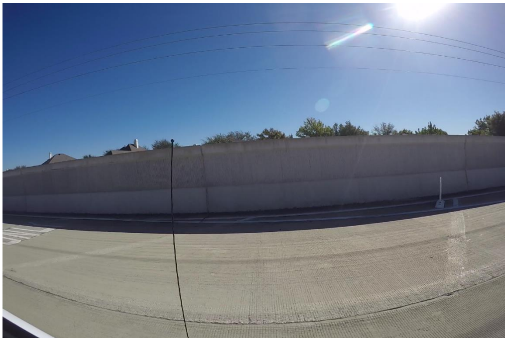
Figure 3.13 Northbound frontage road. Minor spalling of the longitudinal joint as recorded by video
