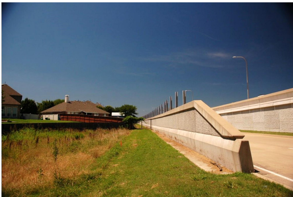
Figure 7.15 Noise wall installation progress on the west side. Sloped southernmost end of the wall (June 13, 2019)
