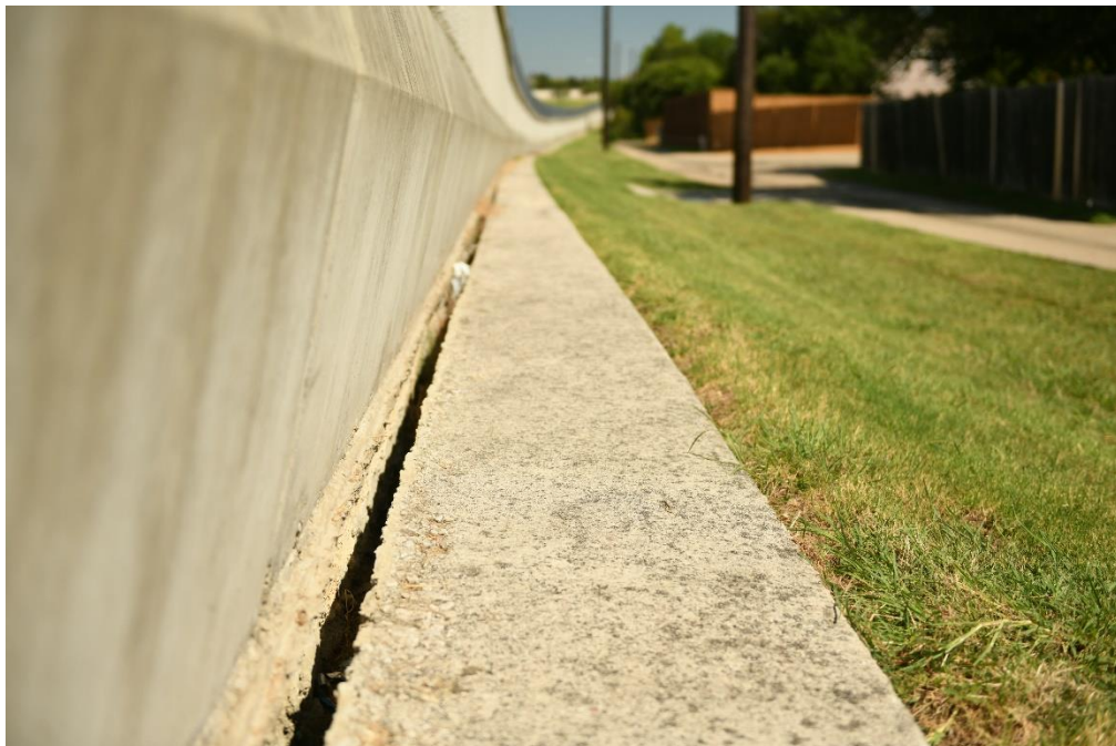
Figure 7.38 Separation between noise wall and concrete base, east side wall, close to receiver R#1
