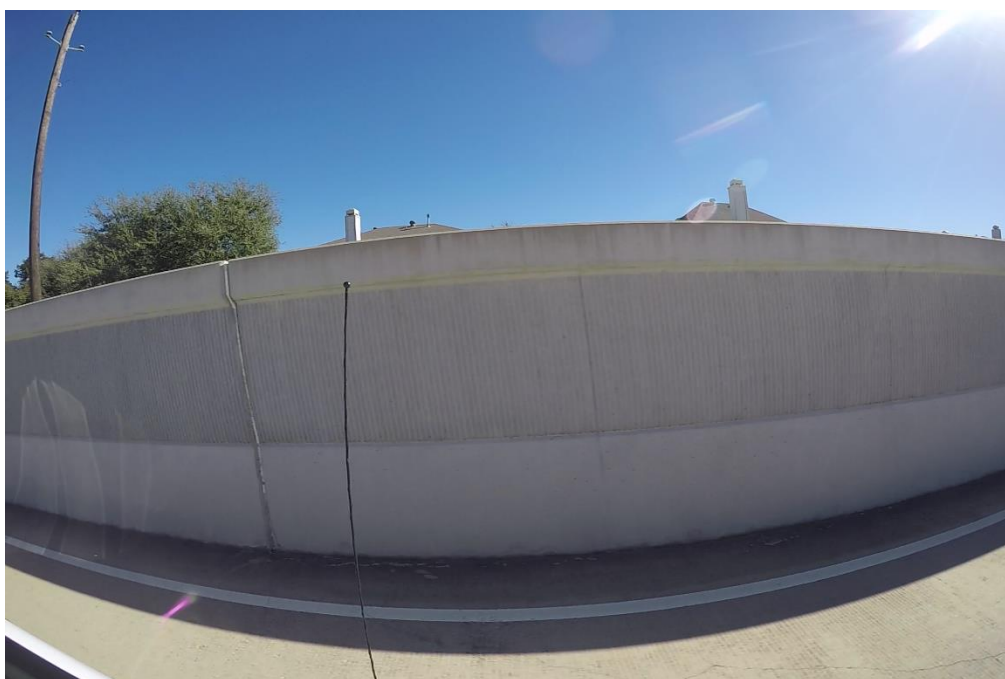
Figure 3.12 Northbound frontage road. Longitudinal crack as recorded by video
