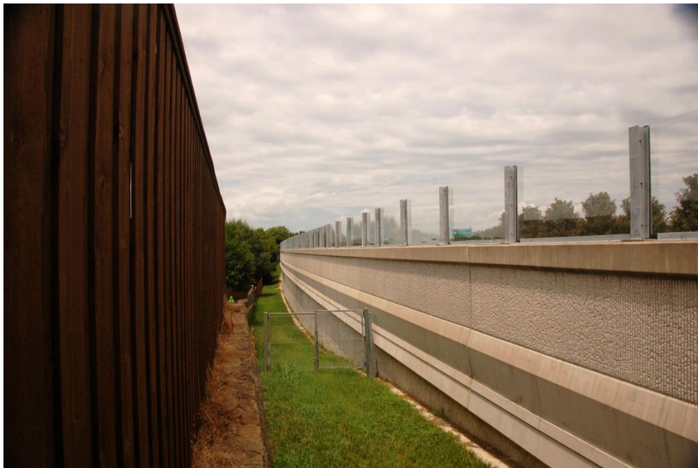
Figure 7.31 West side noise wall finalized, as seen from the neighborhood side (August 14, 2019)
