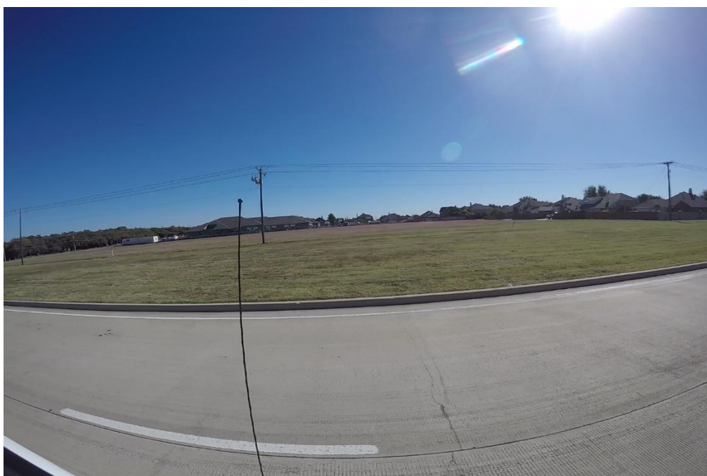
Figure 3.14 Northbound frontage road. Minor spalling of the transverse crack as recorded by video
