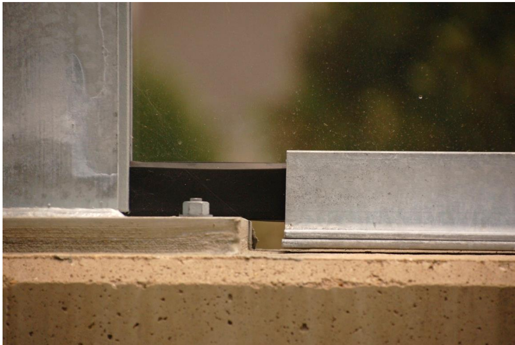
Figure 7.29 Gap and opening; west side noise wall finalized, as seen from the neighborhood side (August 14, 2019)
