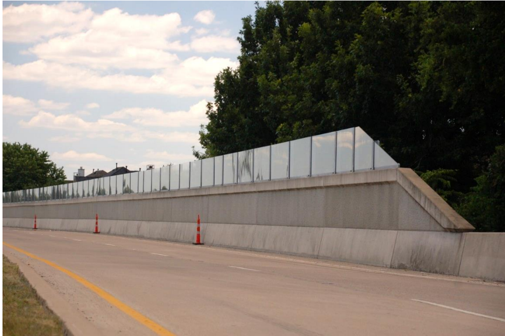
Figure 7.16 Northernmost end of the west side wall near Kirby Road, with the wall near completion (July 24, 2019)
