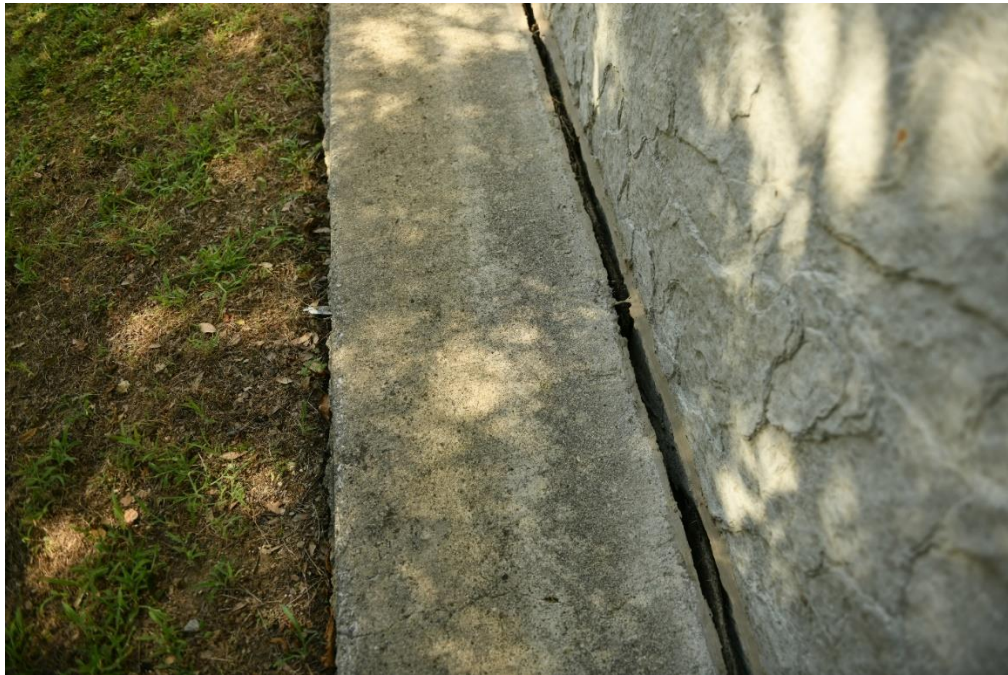
Figure 7.40 Separation between noise wall and concrete base, west side wall, close to receiver R#12
