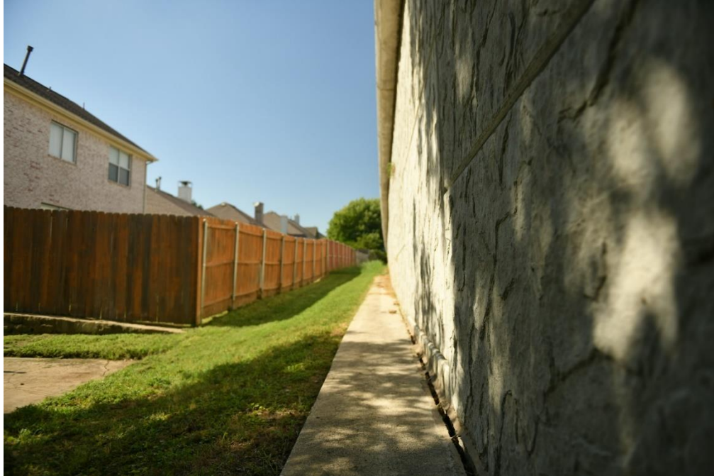
Figure 7.41 Separation between noise wall and concrete base, west side wall, close to receiver R#12
