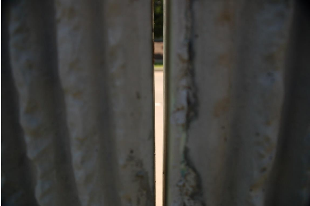
Figure 7.35 Open expansion joint without sealant material
