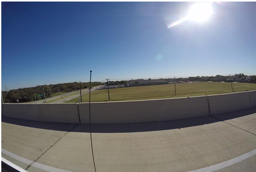
Figure 3.19 Northbound main lane. Expansion joints in the elevated section as recorded by video
