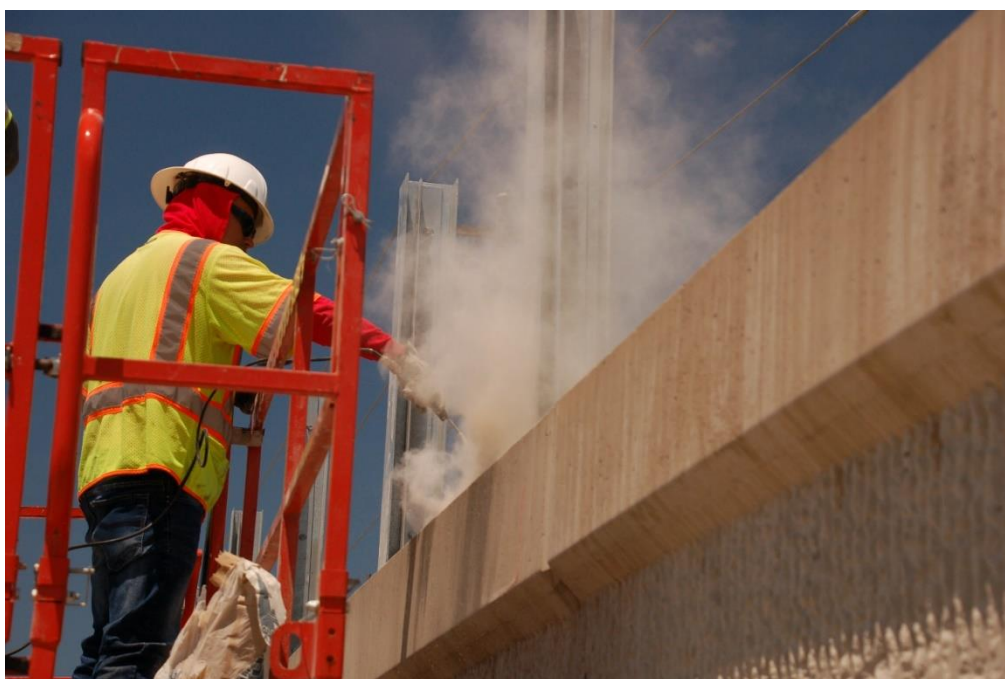
Figure 7.26 East side noise wall installation. A crew member cleans the concrete after the drilling process (July 24, 2019)
