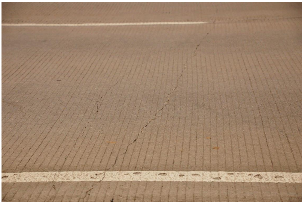
Figure 3.11 Northbound frontage road. Transverse cracks
