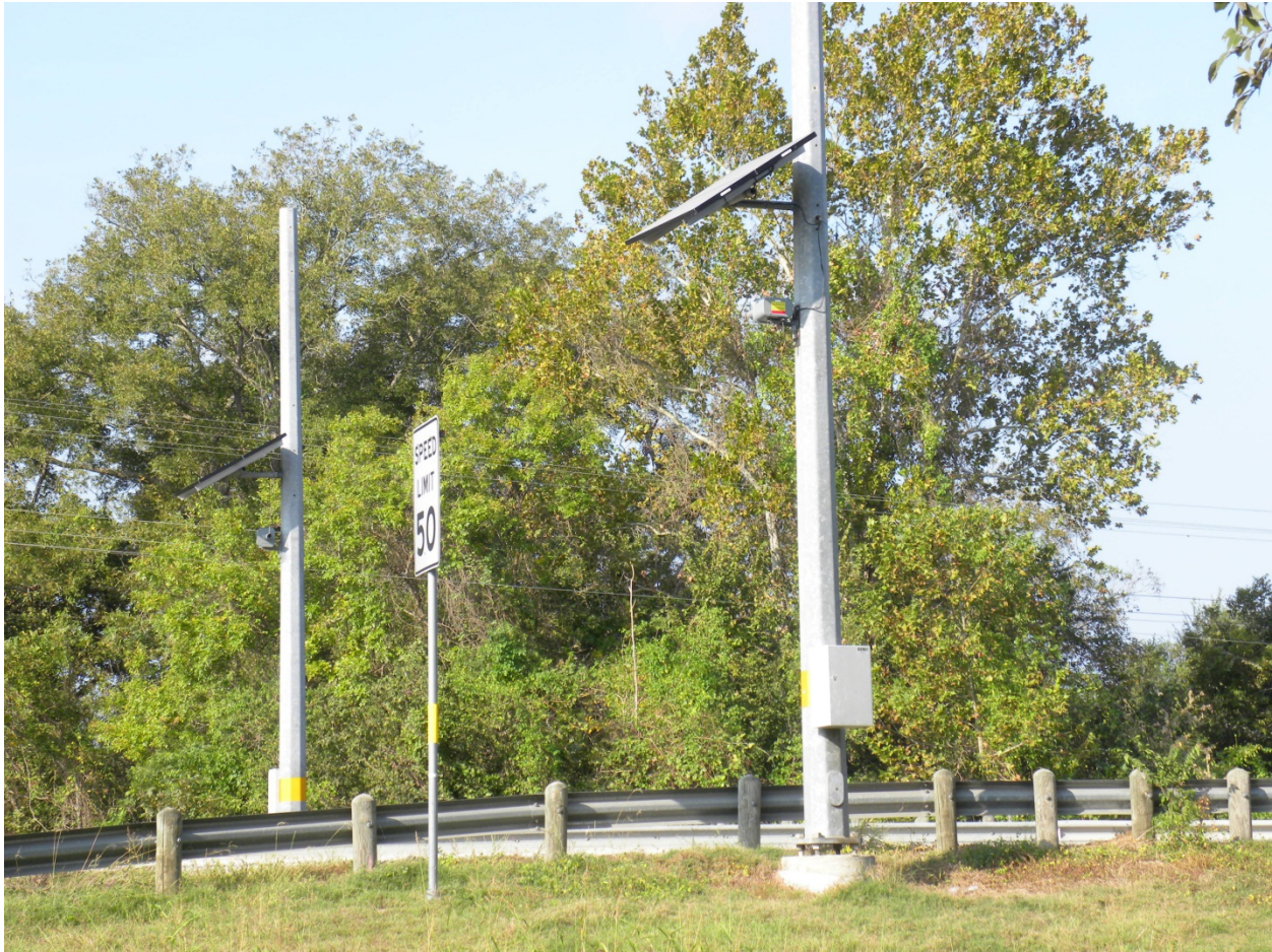
Figure 4.32: Overheight Load Detection Device—Yoakum District (ELTEC 2012)
