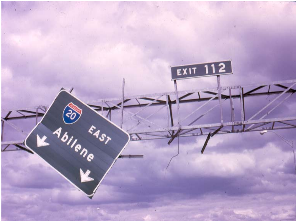
Figure 1.9: Damage to Sign on IH 20 in Abilene District
