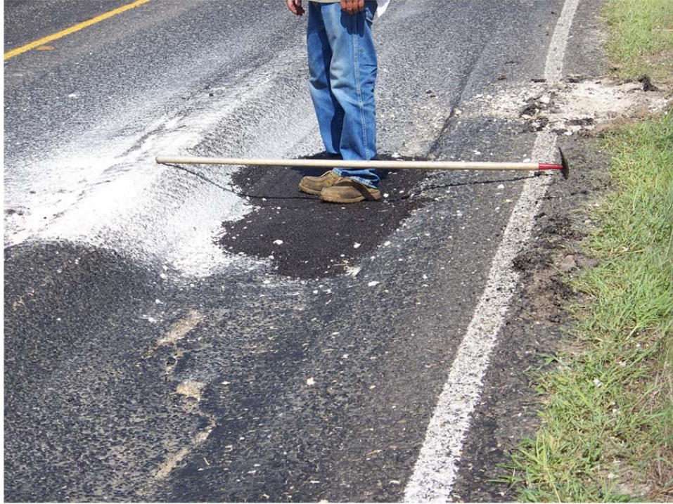
Figure 4.19: Severe Rutting and Shoving Due to Heavy Axle Loads from Three-Axle Farm Trucks
