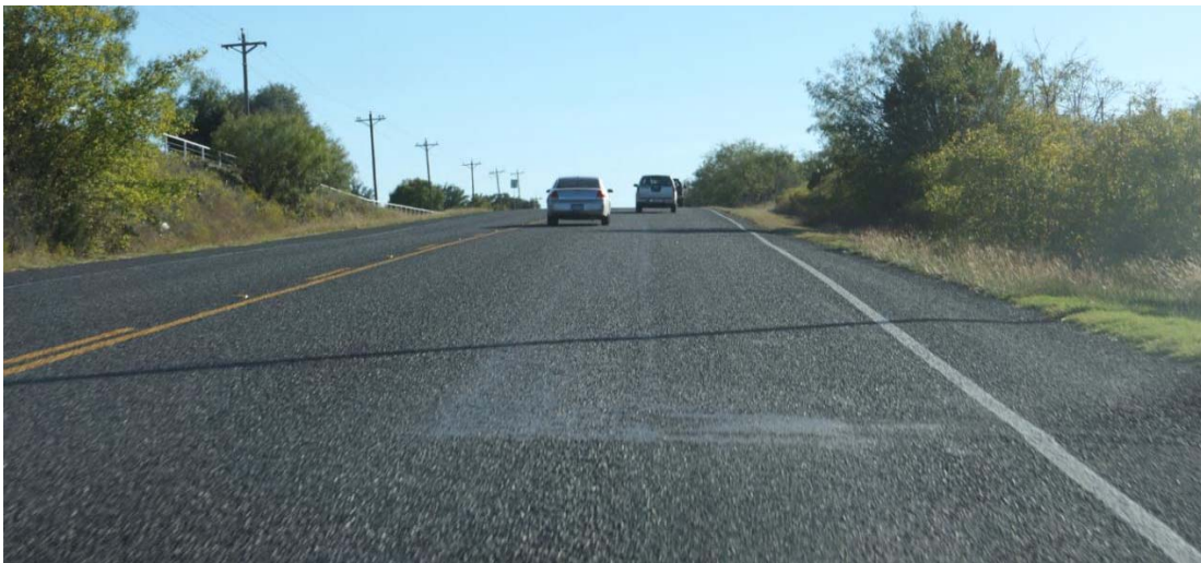
Figure 4.26: Extra-Wide Lane within Transition from One to Two Lanes on “Super 2” Route on US 281
