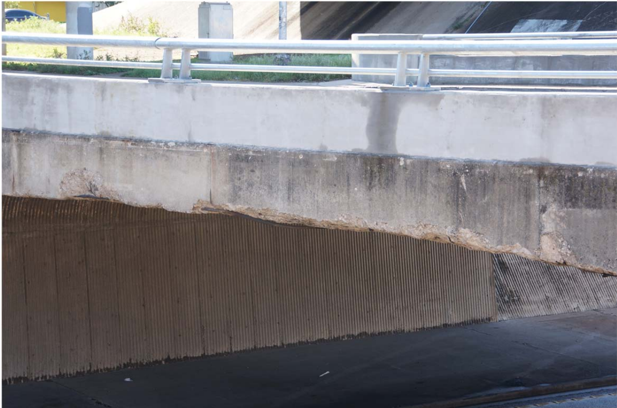
Figure 4.33: Concrete Spalling and Exposed Rebar Attest to Several OS/OW Hits—Austin District
