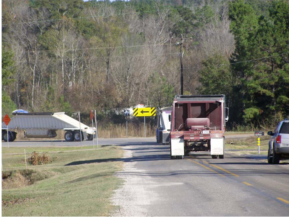
Figure 4.21: Heavy Trucks Operating along a Narrow FM Road and Resulting Pavement Deformation
