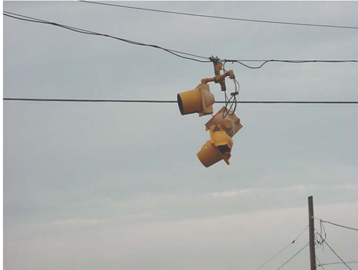
Figure 1.10: Damaged Traffic Signal
