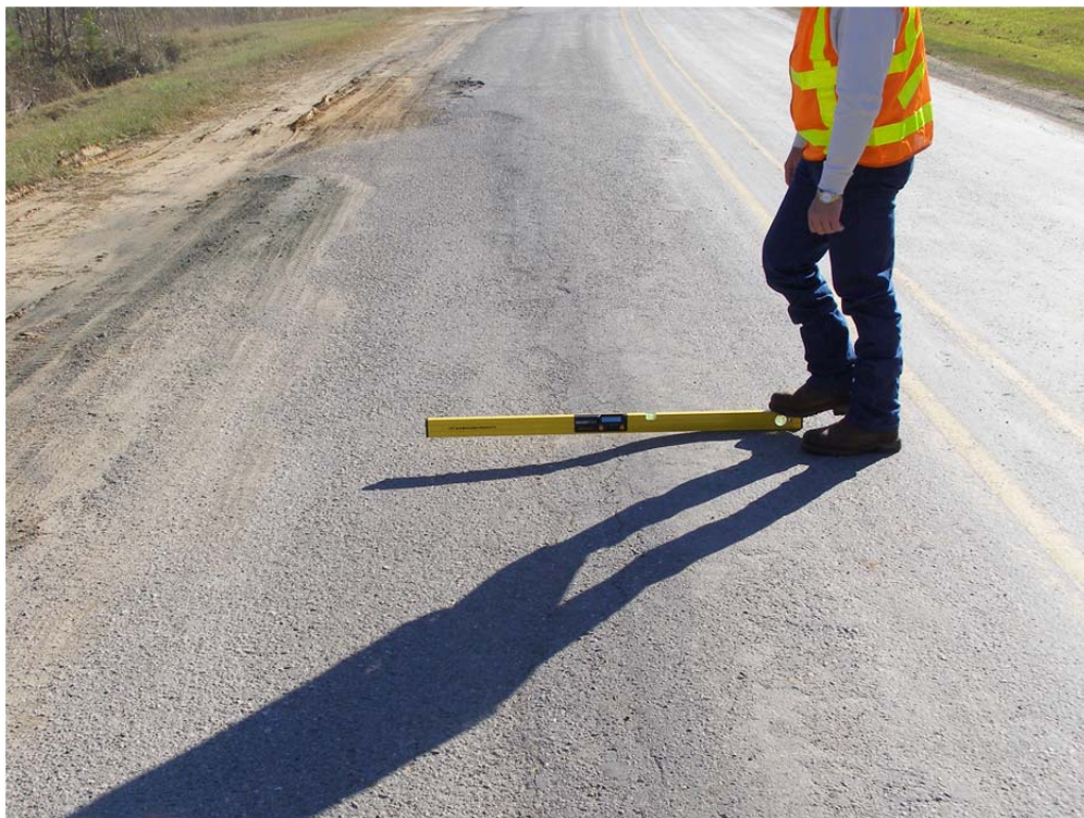
Figure 4.22: Excessive Surface Deformation from Heavy Wheel Loads near the Pavement Edge
