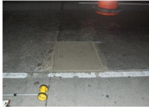
Small PCC patch
