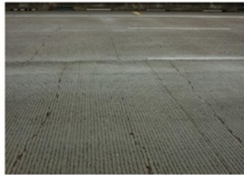
Closely spaced transverse cracks
