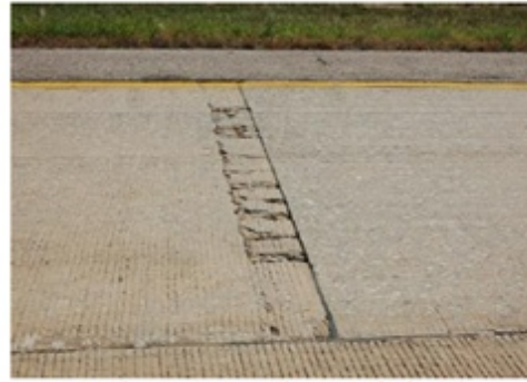
Punchout at joint (SB inside lane)
