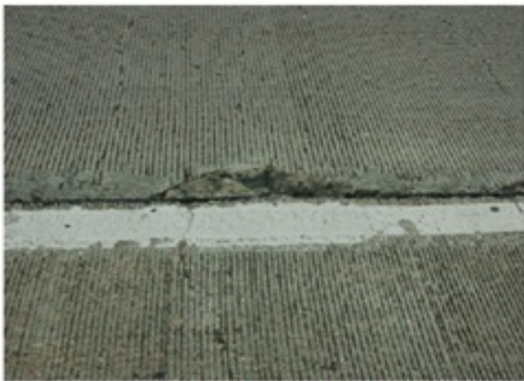
Longitudinal joint damage
