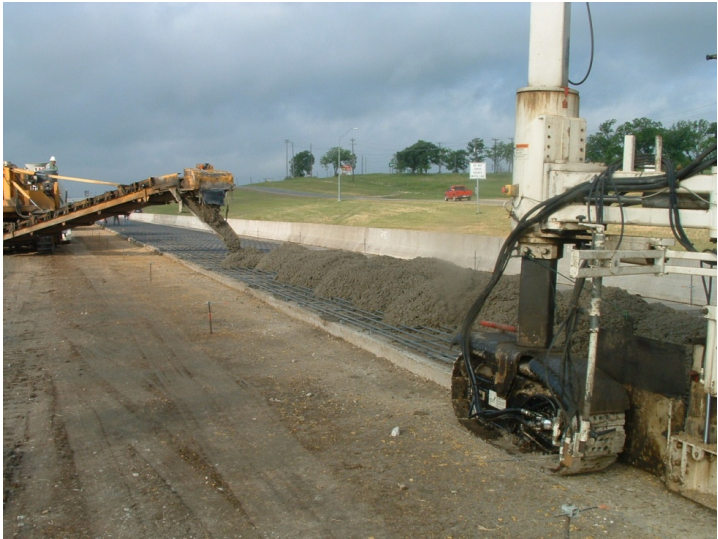
Figure 3.10: Concrete too far ahead of the paving machine
