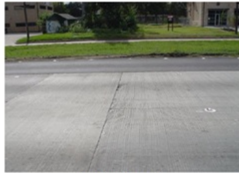
Patch with spall
