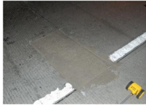
Small PCC patch
