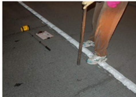
Sounding of delaminated area with no superficial distresses
