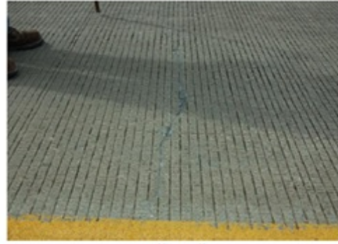
Small spalls 1989-1990 Experimental sections (EB)
