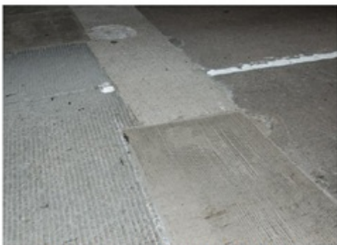
Patches at eastbound end of BCO
