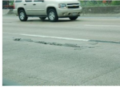
AC Patch, longitudinal cracks
