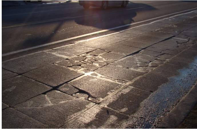
Figure 2.10: Failed joints in wheel path
