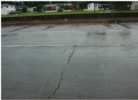
Wide transverse crack
