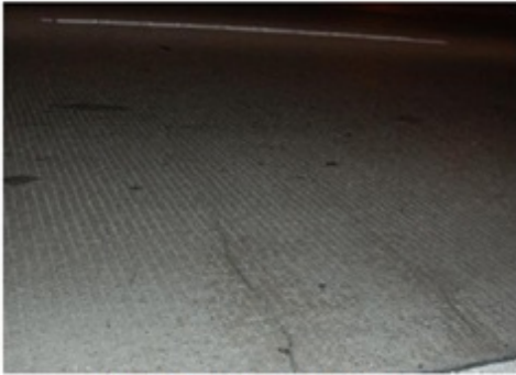
Typical transverse cracks
