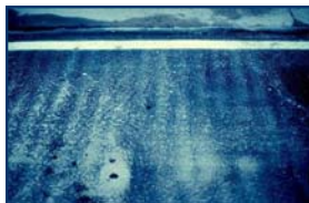
Over or Under-Compaction Can Occur
