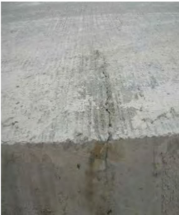
Figure 2.14: (a) Large crack width on the surface
