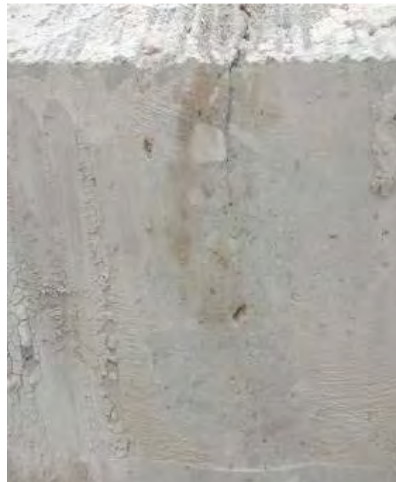
Figure 2.14: (b) Tight crack widths
