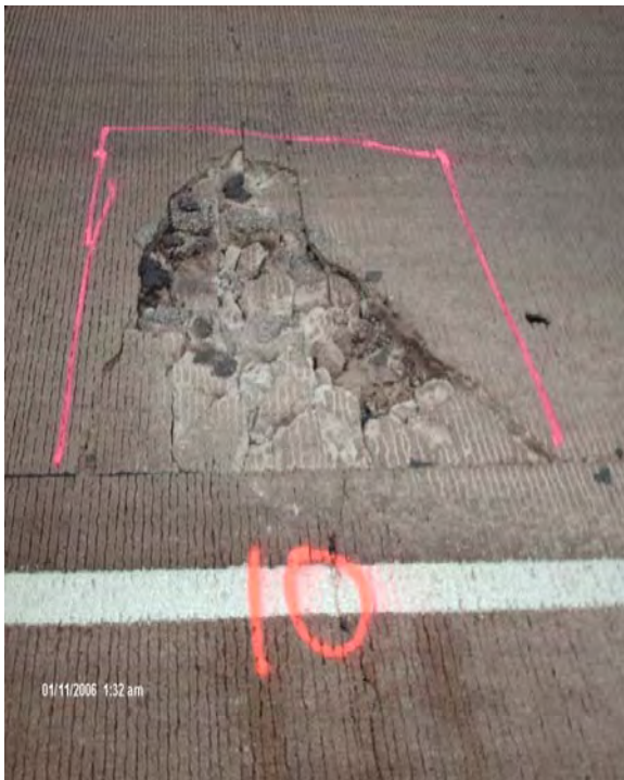
Figure 2.17: Distress due to mid-depth horizontal cracking
