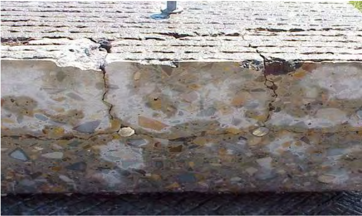
Figure 2.16: Slab segment showing horizontal cracking at the mid-depth, longitudinal crack above longitudinal steel, and sound concrete at the bottom half
