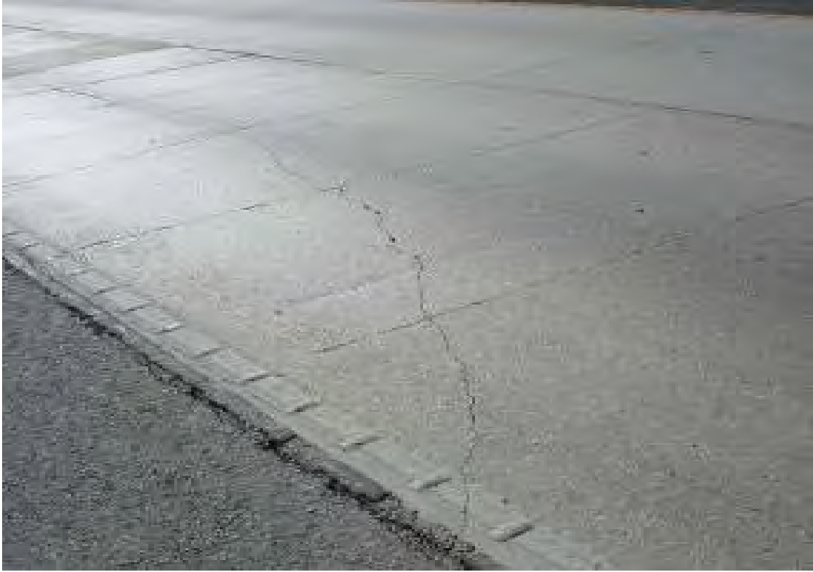
Figure 2.21: Half moon shape longitudinal crack
