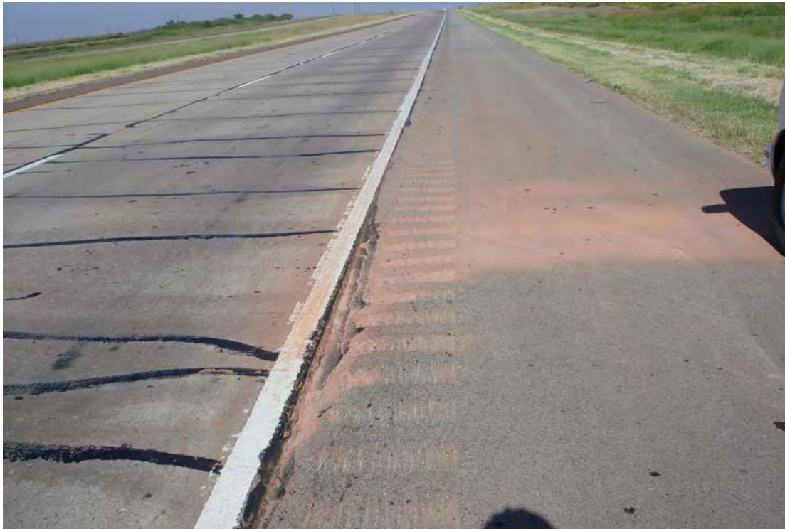
Figure 2.20: CRCP with severe pumping
