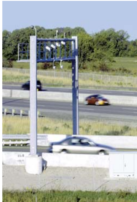
Figure 2.1: Toll Tag Reader
