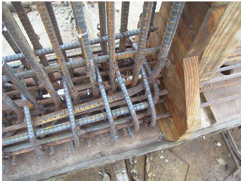
Figure 9.3 Reinforcement Congestion in End Region Bottom Flange of Type A Beams
