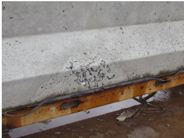
Figure 9.16 Voids at Location of SCC Discharge for First Batch
