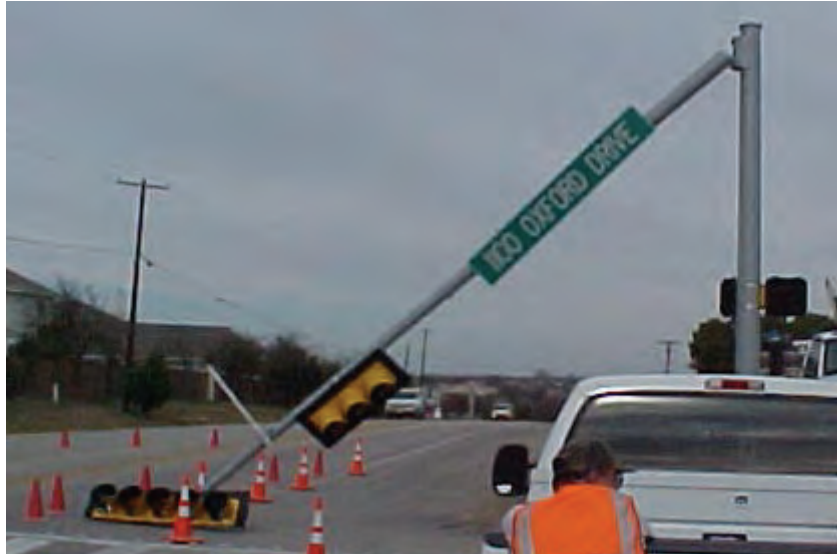
Figure 1.1: Failure of Cantilevered Traffic Signal Structure in Pflugerville, Texas in December 2003
