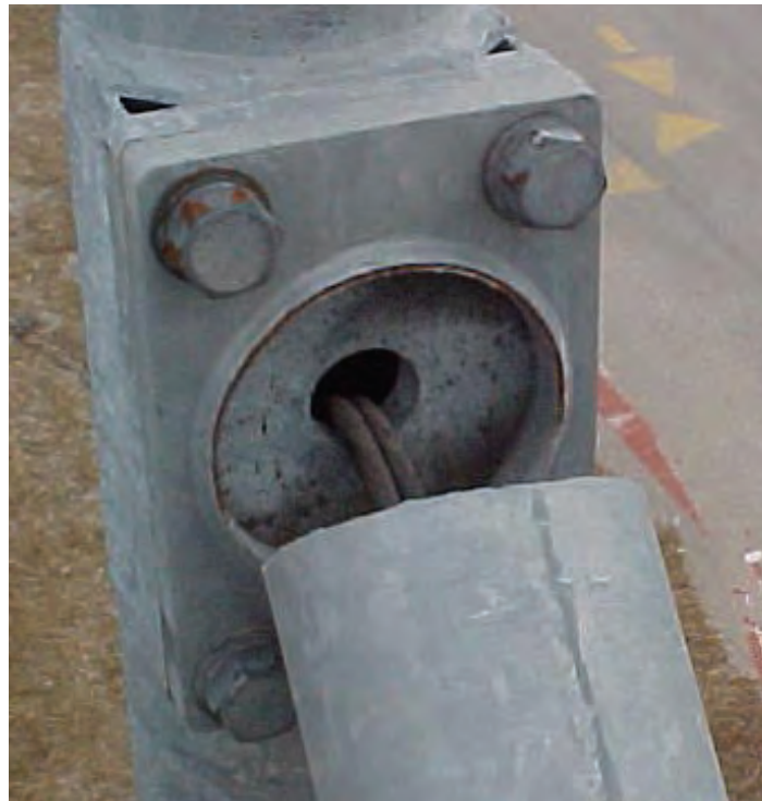
Figure 1.2: Fatigue Crack Initiated by Cyclic Loading
