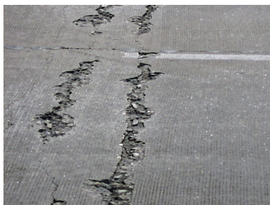
Figure 1 – Severe Spalling of CRCP (Won, 2001)
