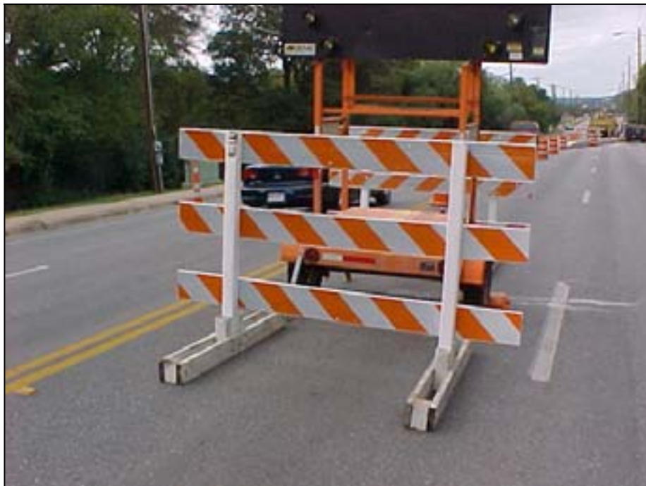
Photo C.4 Barricade installed backside to traffic and too close to arrow board
