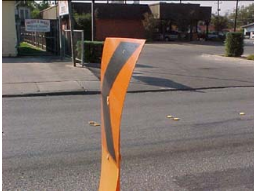
Photo C.17 Typical damage of chevrons
