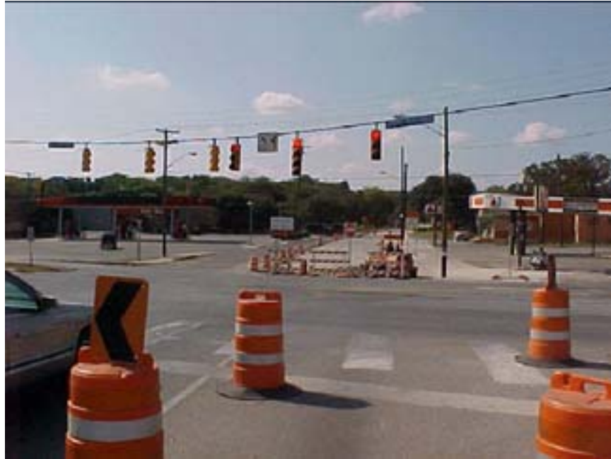
Photo B.19 San Antonio, Work Zone #17, Rittiman Rd.: View of work zone initial section at Harry Wurzbach
