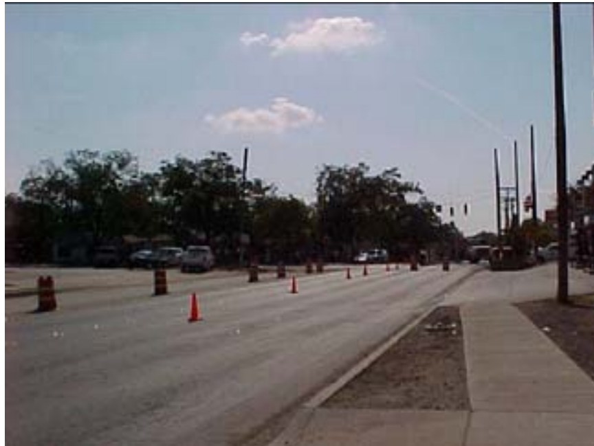
Photo B.17 San Antonio, Work Zone #16, Probandt and Mitchell St.: General view of work zone on Probandt St.
