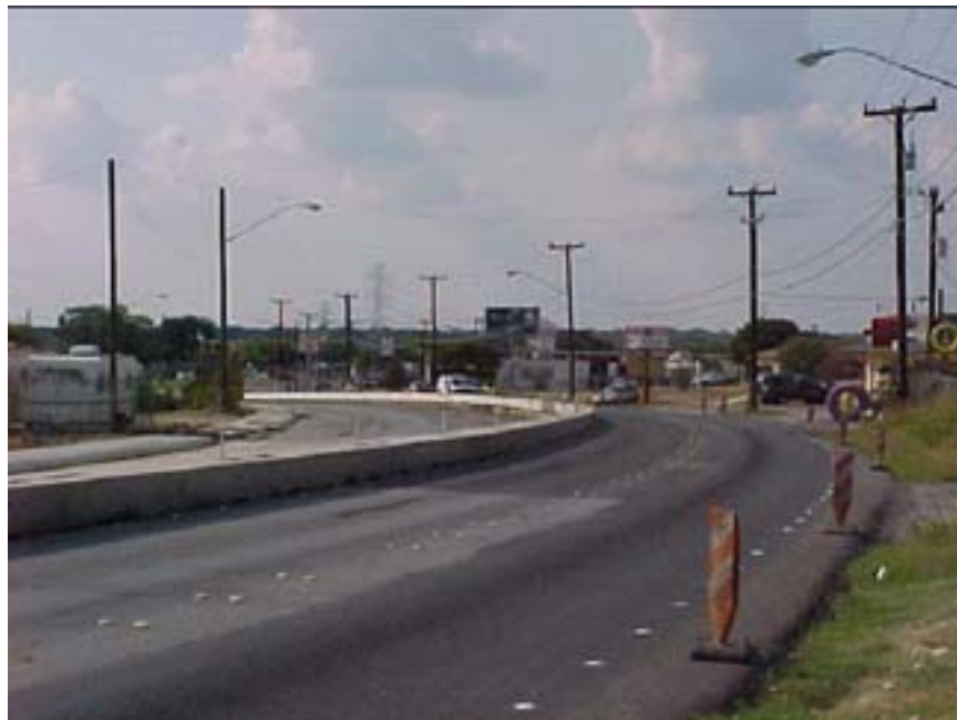
Photo B.26 San Antonio, Work Zone #18, O'Connor Rd.: View of work zone main section, facing northwest
