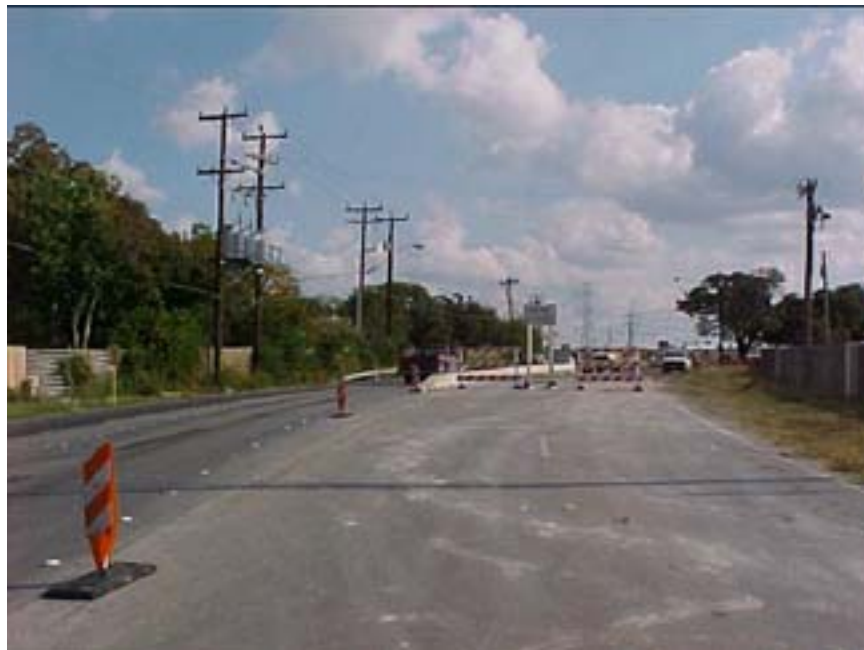
Photo B.24 San Antonio, Work Zone #18, O'Connor Rd.: View of work zone northwest initial section
