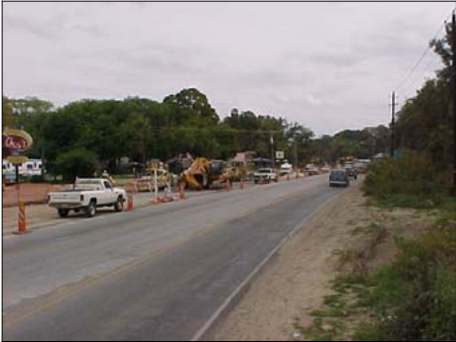
Photo A.14 Austin, Work Zone #5, Barton Springs Rd.: View of the main construction activity section
