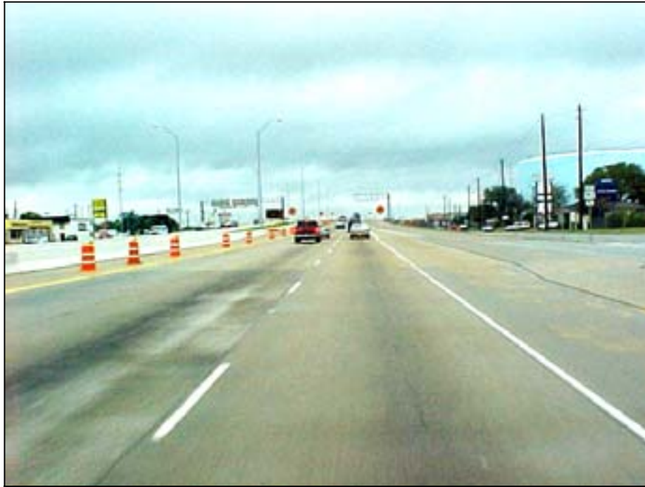
Photo A.23 Austin, Work Zone #9, Research Blvd.: View of northbound work zone initial section
