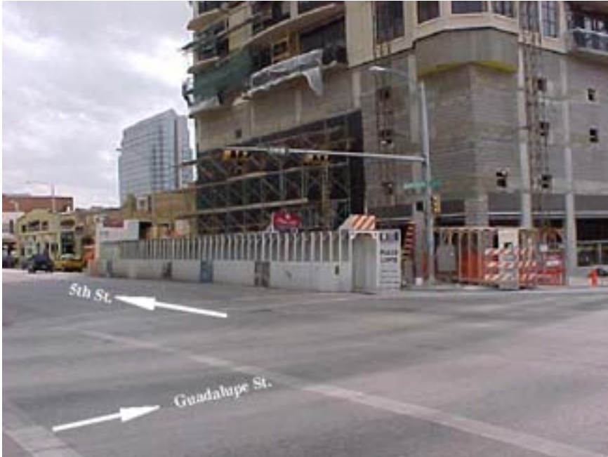
Photo A.7 Austin, Work Zone #3, 400 Guadalupe St.: General view of work zone section on 5 th Street
