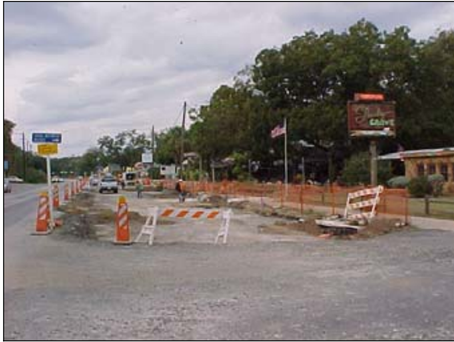
Photo A.15 Austin, Work Zone #5, Barton Springs Rd.: View of the main construction activity section
