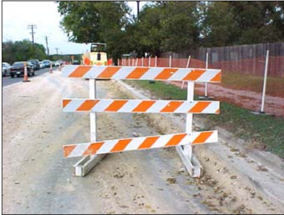
Photo C.7 Insufficient barricade assembling
