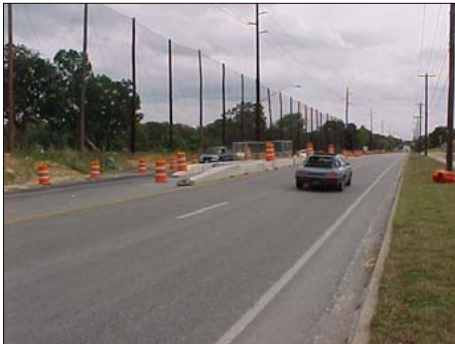
Photo A.10 Austin, Work Zone #4, Lake Austin Blvd.: General view of the main construction area from eastbound
