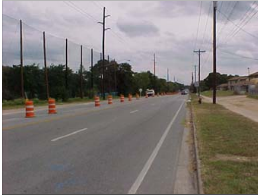
Photo A.11 Austin, Work Zone #4, Lake Austin Blvd.: Work zone initial section (eastbound)
