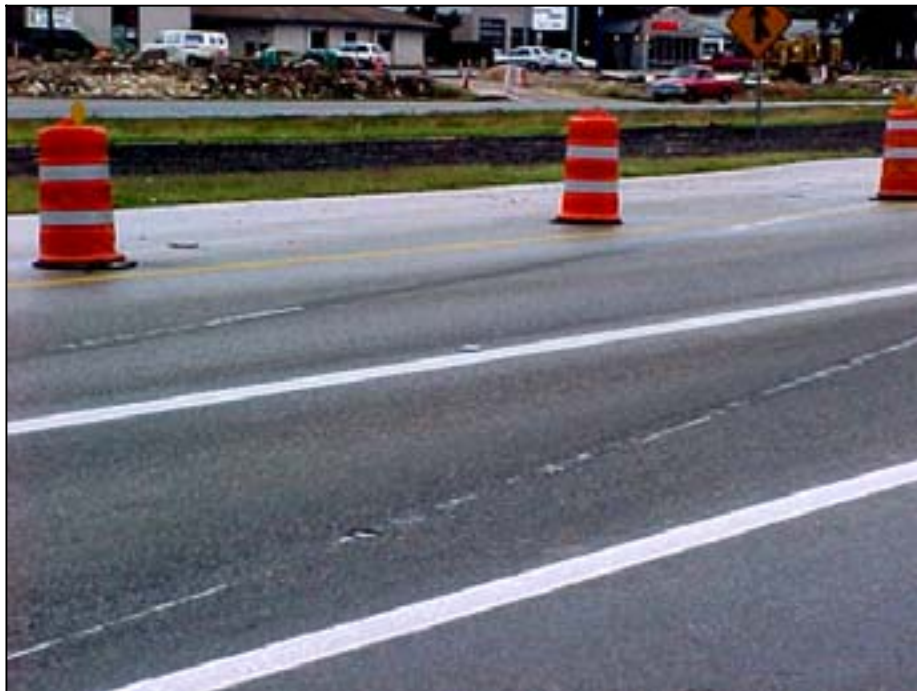
Photo C.12 Old pavement stripes were not completely removed
