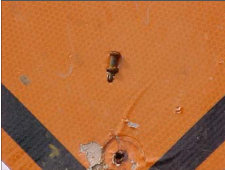
Photo C.1 Insufficient condition of sign. Sign fastened to support with nails.
