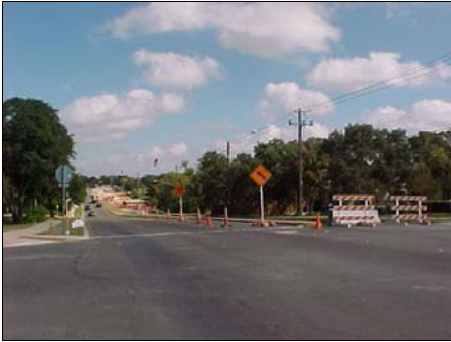
Photo A.19 Austin, Work Zone #7, Amherst Dr.: General view of work zone
