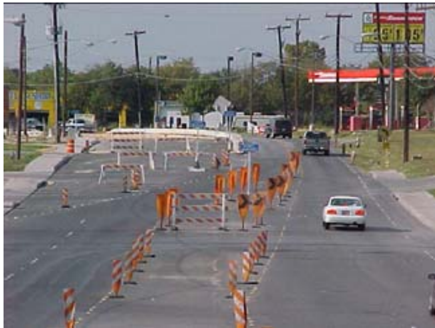
Photo B.28 San Antonio, Work Zone #18, O'Connor Rd.: View of work zone southeast initial section (at IH 35)
