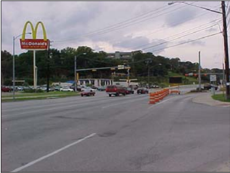
Photo A.13 Austin, Work Zone #5, Barton Springs Rd.: View of east end of work zone
