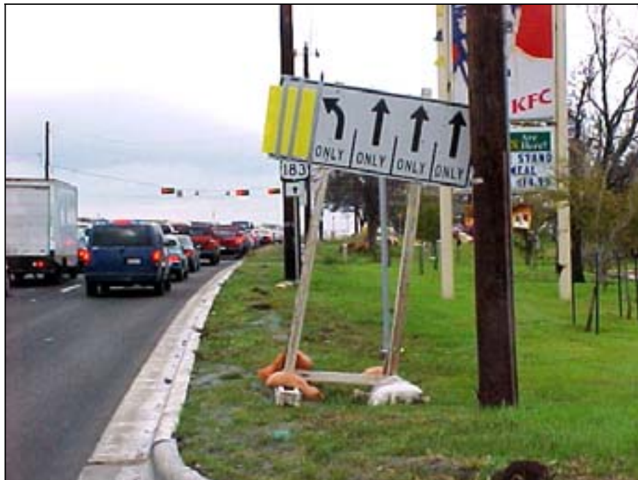
Photo C.14 Insufficient signs installation
