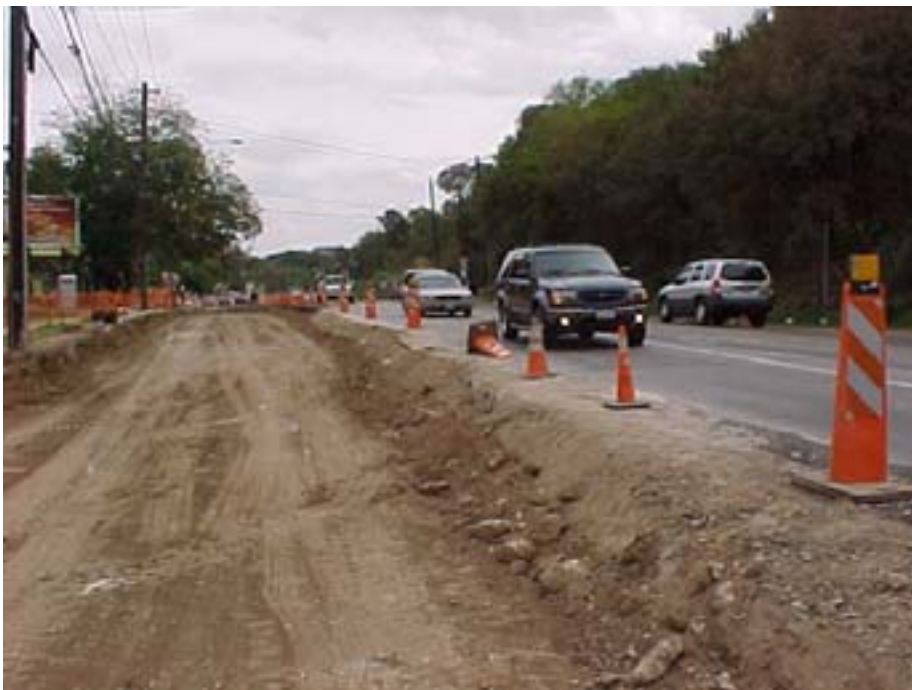
Photo C.6 Pavement drop off
