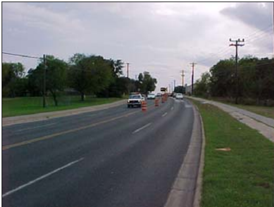
Photo A.16 Austin, Work Zone #6, Manchaca Rd.: View of northwest end of work zone
