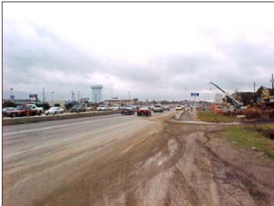
Photo A.30 Austin, Work Zone #9, Research Blvd.: Southbound view between Lake Creek Pkwy. and Anderson Mill Rd.
