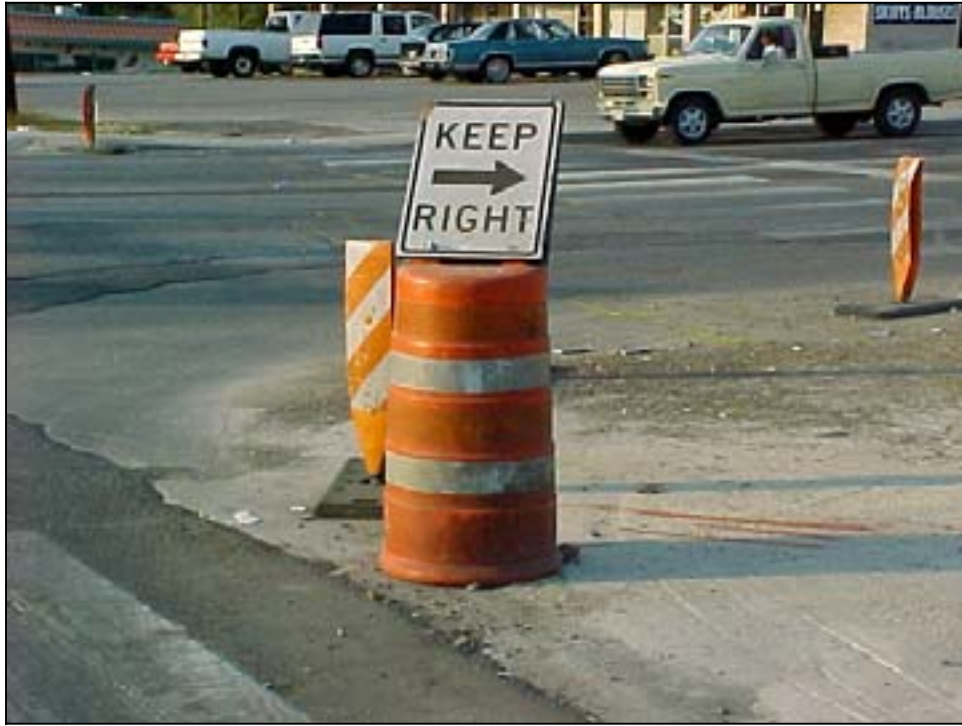
Photo C.21 A plywood "Keep Right" sign not approved to be attached to a plastic drum
