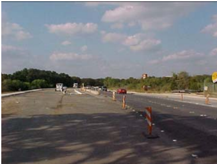
Photo B.12 San Antonio, Work Zone #14, FM 2696: Work zone view between Bitters Rd. and Lariat St.
