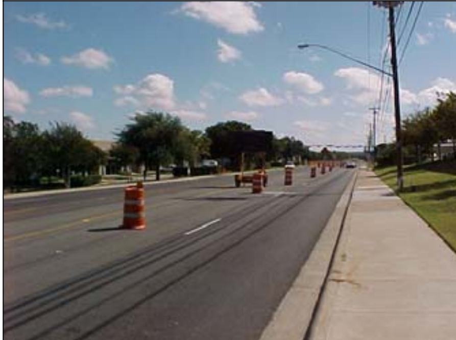
Photo A.20 Austin, Work Zone #8, Rutland Dr.: View of the east end of work zone
