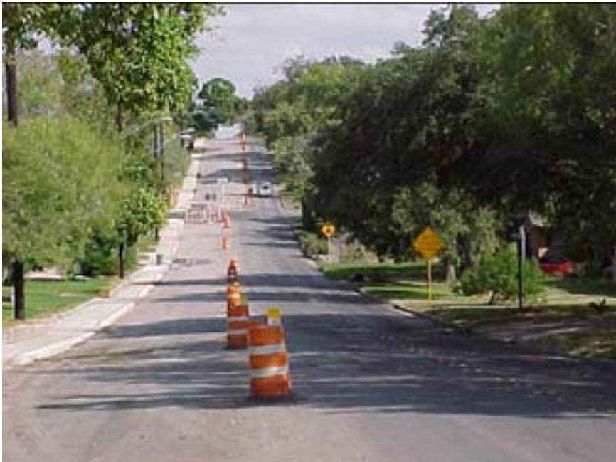
Photo B.21 San Antonio, Work Zone #17, Rittiman Rd.: Two-way road to one-way road transition section at N. Vandiver intersection
