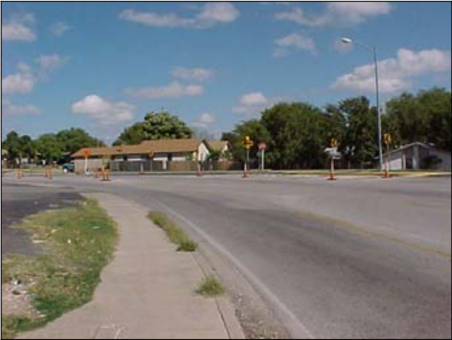
Photo A.21 Austin, Work Zone #8, Rutland Dr.: View of the west end of work zone
