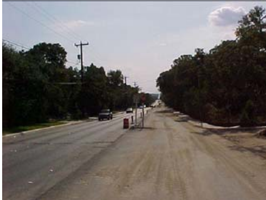
Photo B.9 San Antonio, Work Zone #13, West Ave.: General view of work zone
