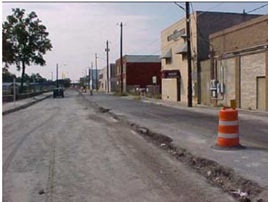
Photo C.18 Example of Pavement Drop-Off and Excessive Distance between Drums
