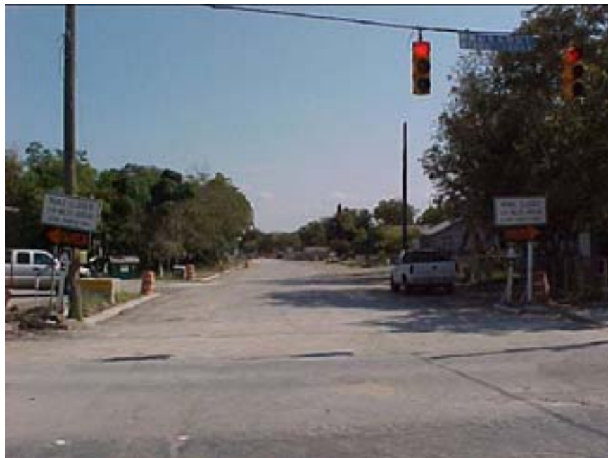
Photo B.18 San Antonio, Work Zone #16, Probandt and Mitchell St.: General view of work zone on Mitchell St.
