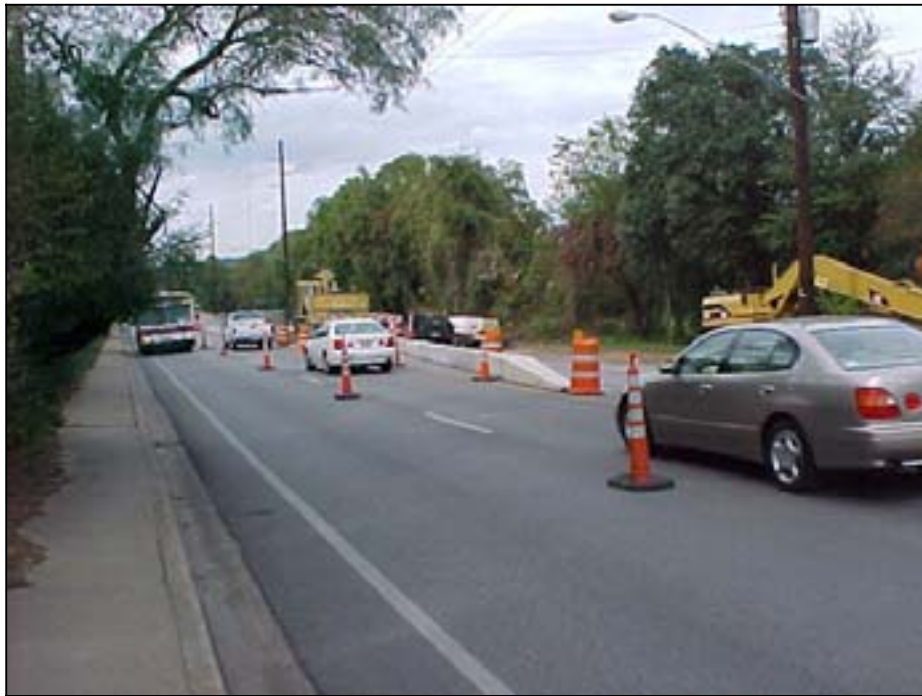
Photo A.9 Austin, Work Zone #4, Lake Austin Blvd.: General view of the main construction area
