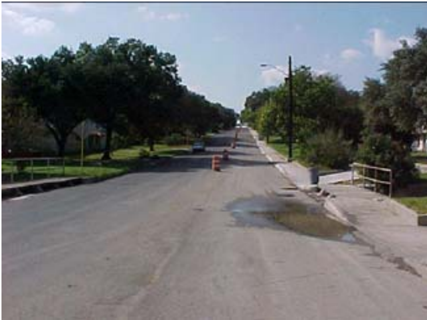
Photo B.22 San Antonio, Work Zone #17, Rittiman Rd.: Work zone view between N. Vandiver and Loop 368
