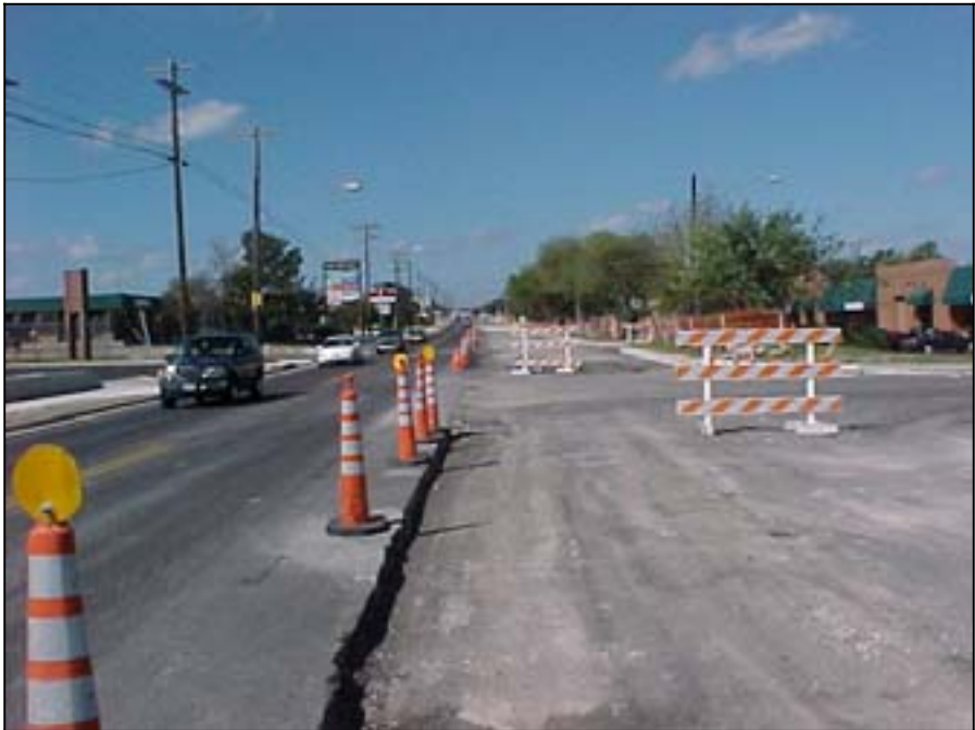
Photo A.22 Austin, Work Zone #8, Rutland Dr.: View of the main construction activity section
