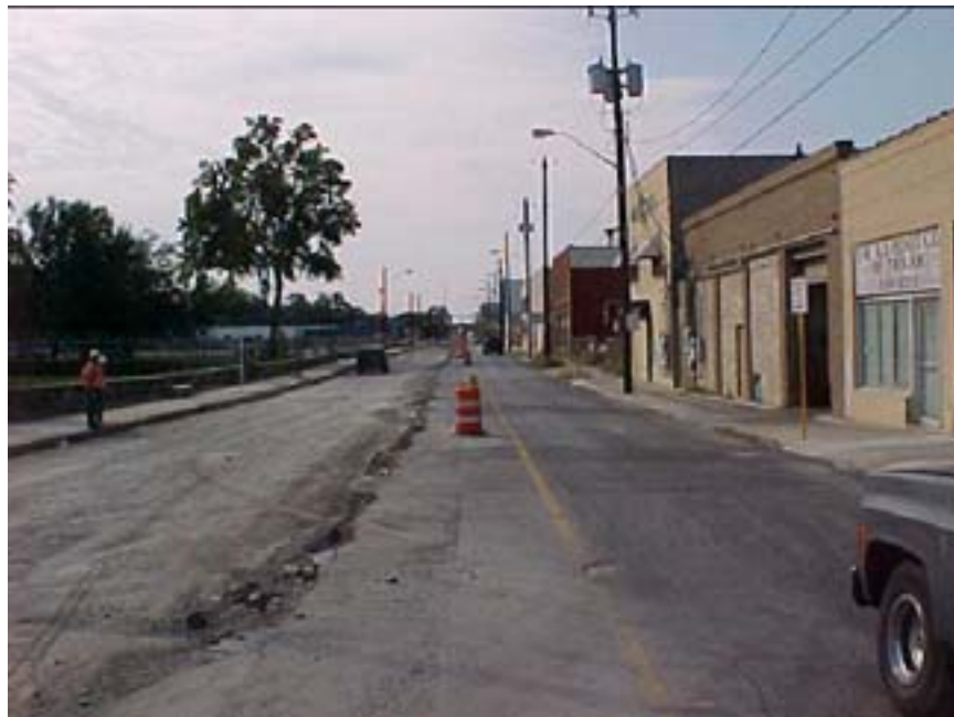
Photo B.2 San Antonio, Work Zone #11, S. Flores St.: General view of the work zone
