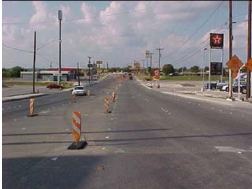
Photo B.27 San Antonio, Work Zone #18, O'Connor Rd.: View of work zone southeast initial section (at IH 35)
