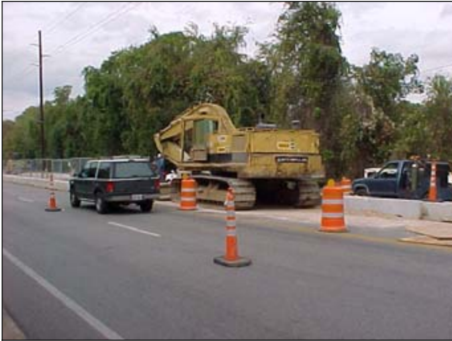
Photo C.5 Construction mechanism too close to traffic
