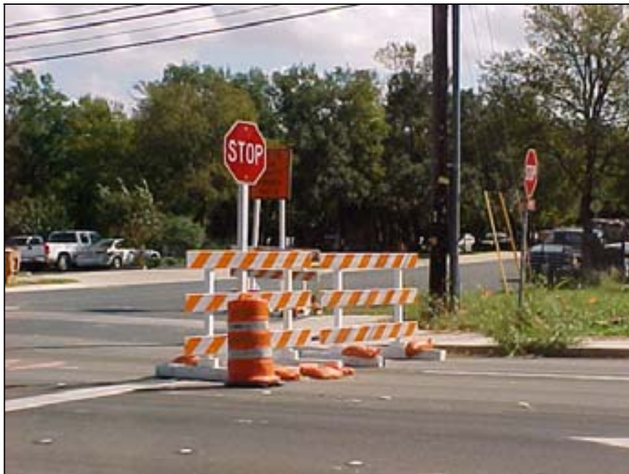
Photo C.8 Sign and barricade do not have the required 10-foot buffer space
