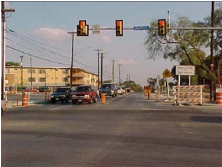
Photo B.16 San Antonio, Work Zone #15, Blanco–Jackson Keller Intersection: Westbound approach (Jackson Keller Rd.), facing east
