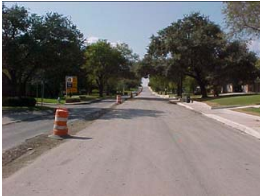
Photo B.20 San Antonio, Work Zone #17, Rittiman Rd.: Work zone view between Harry Wurzbach and N. Vandiver
