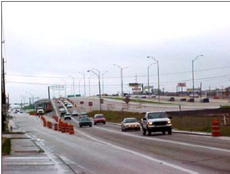
Photo A.24 Austin, Work Zone #9, Research Blvd.: Initial section of northbound detour
