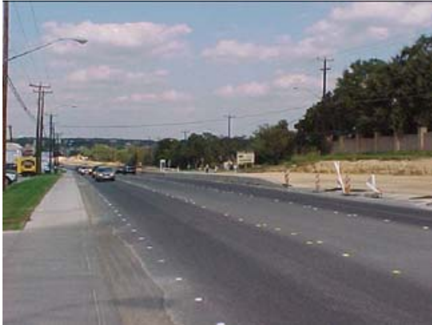
Photo B.11 San Antonio, Work Zone #14, FM 2696: Work zone view between Vista Real and Bitters Rd.
