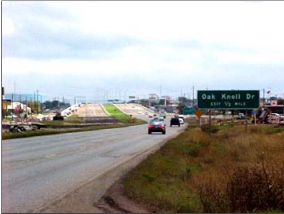
Photo A.33 Austin, Work Zone #9, Research Blvd.: View of work zone south end
