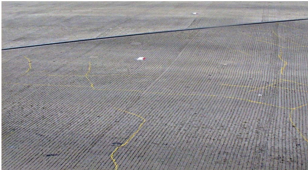
Figure 4.3 Stair-step Cracking on the Dow Bridge near Expansion Joint
