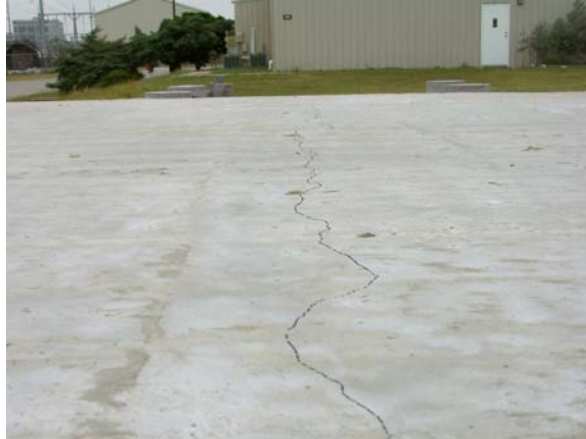
Figure 5.19 Photograph of drying shrinkage cracking on HPC Phase I LSBDD after eight days. Crack is outlined in black for visual reference
