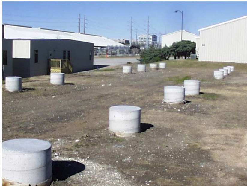
Figure 5.6 Photograph of poured columns used to prevent differential settlement of the LSBDs
