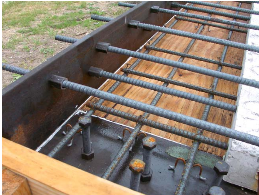
Figure 5.9 Photograph of the end region showing two layers of threaded reinforcing bar as well as a bottom layer of deformed reinforcing bar
