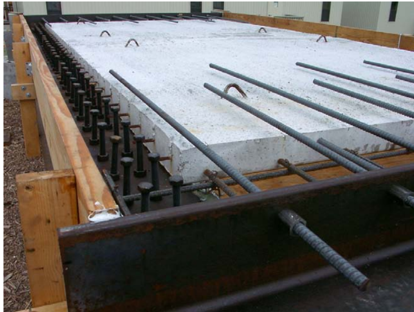
Figure 5.8 Photograph of shear studs a day before the cast-in-place concrete was poured
