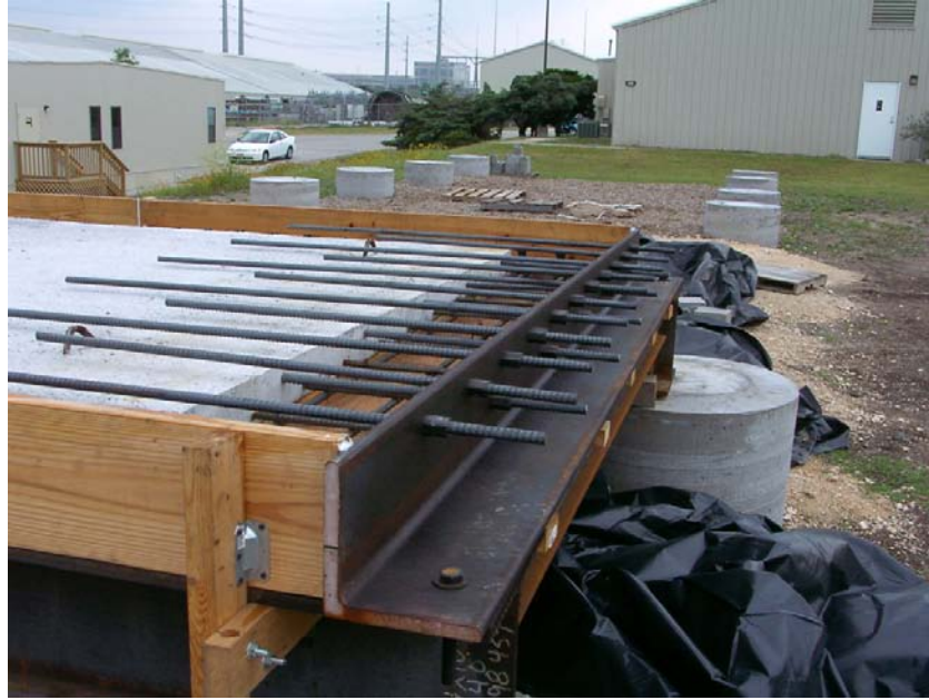
Figure 5.10 Photograph of 8 in. x 8 in. steel angle. The steel angle is bolted to the steel girder to provide a source of high restraint.
