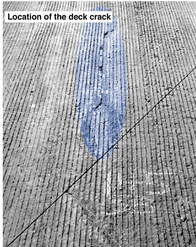
Figure 2.6 Transverse deck crack
