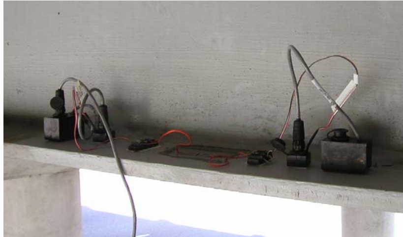
Figure 2.7: MicroSAFE Units Paired on Bridge
