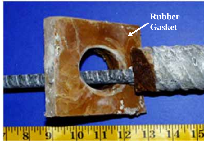
Figure 5.2 Duct Corrosion Found Inside Rubber Gaskets 1
