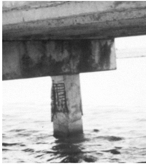
(b) Coastal Saltwater Exposure "Attack from Below"
