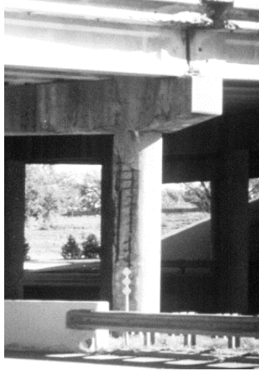
(a) Deicing Chemical Exposure "Attack from Above"
