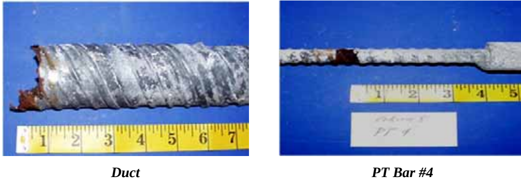
Figure 4.32 Reinforcement Condition for Specimen PT-TC-S-GB 1
