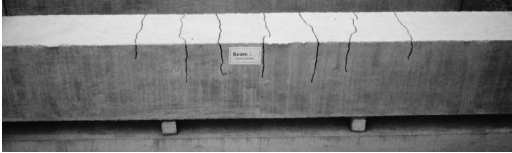
Figure A.43 - Crack Pattern for Specimen 2.9
