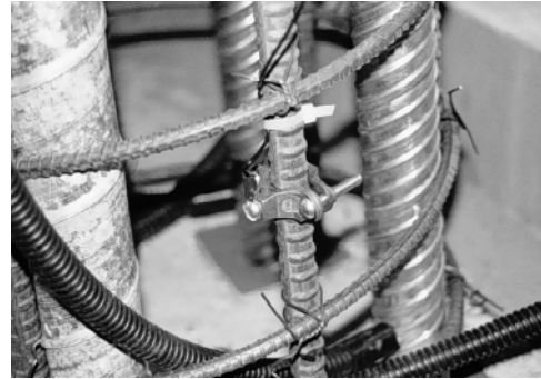
Ground Clamp to Attach Ground Wire
