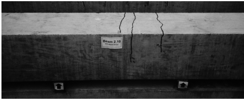
Figure A.44 - Crack Pattern for Specimen 2.10
