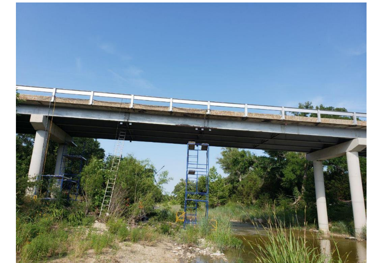
Scaffolding for contact instruments used for validation
