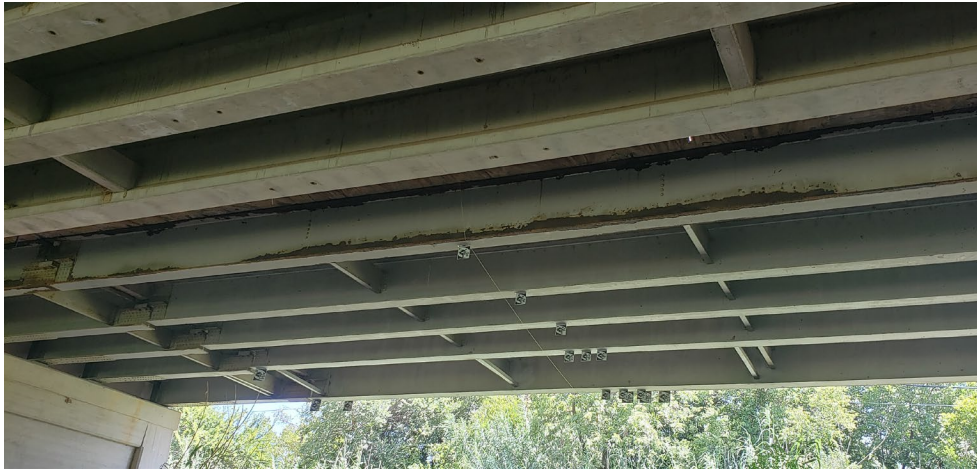
Figure 3-13: attachment of HCPTs to the bridge steel girders.
