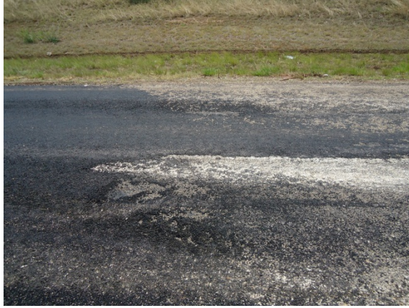
Figure 12. Delamination between the patching mix and existing surface due to poor feathering
