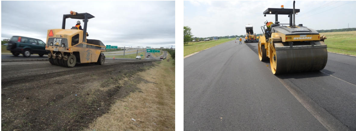
Figure 13. Pneumatic and steel wheel roller compactors used for compacting and smoothing the surface
