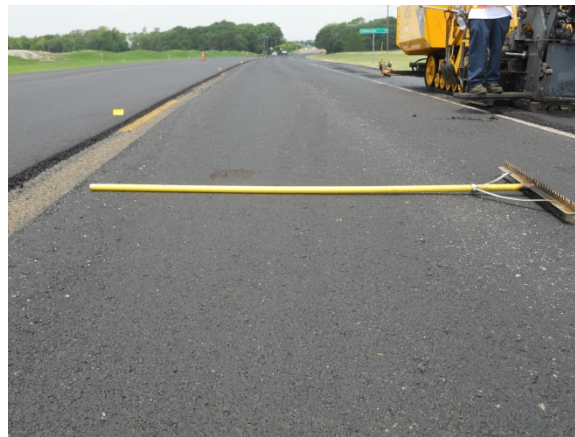
Figure 11. Thin lift level-up mix laid down to establish a base surface for the overlay mix
