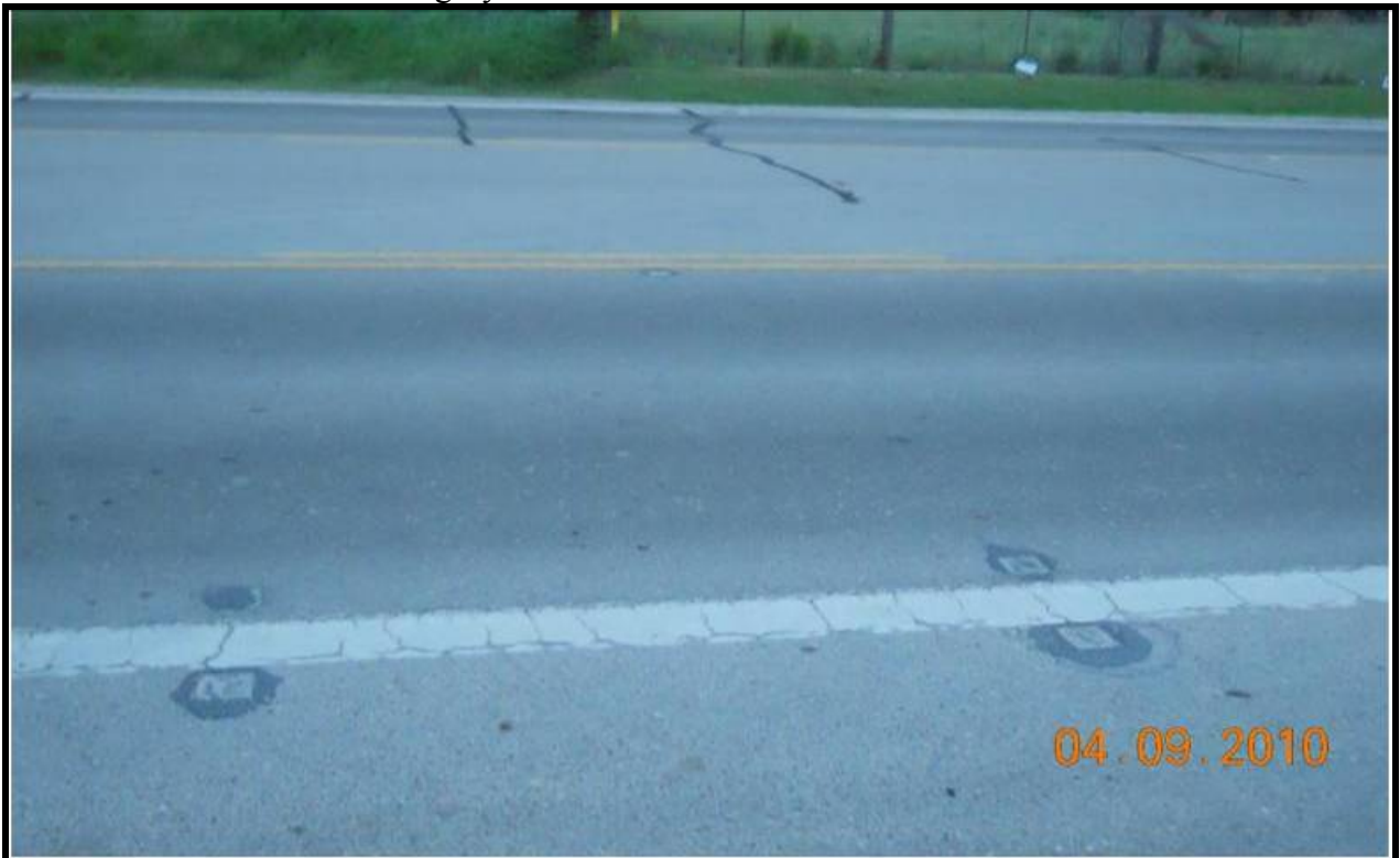
Category 2: FM 907 from SH 107 to FM 1925 (long. and trans. cracking)
