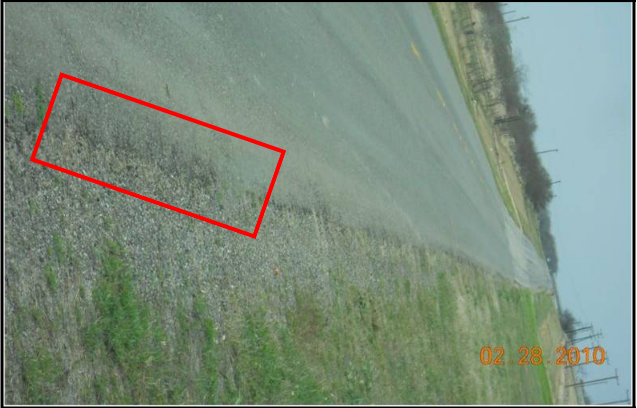
Category 7: FM 624 from SH 359 to US 281 (Edge failure)
