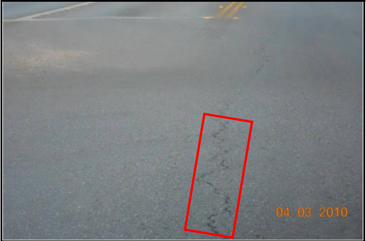
Category 7: FM 758 from Guadalupe county line to FM 78 (long. cracking and raveling)
