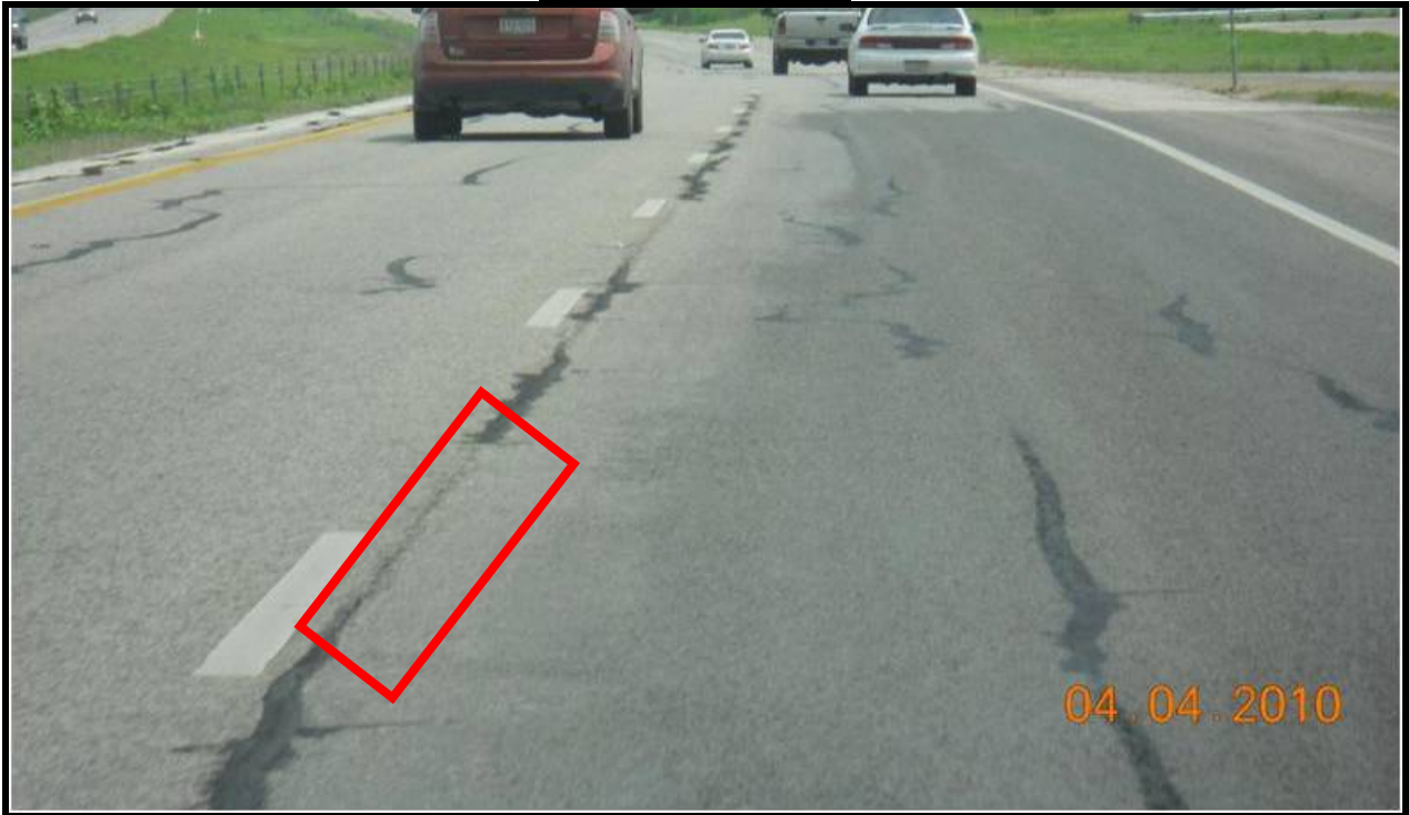
Category 1: US 90 from west of SL 1604 to Bexar county line (long. cracking and poor ride)
