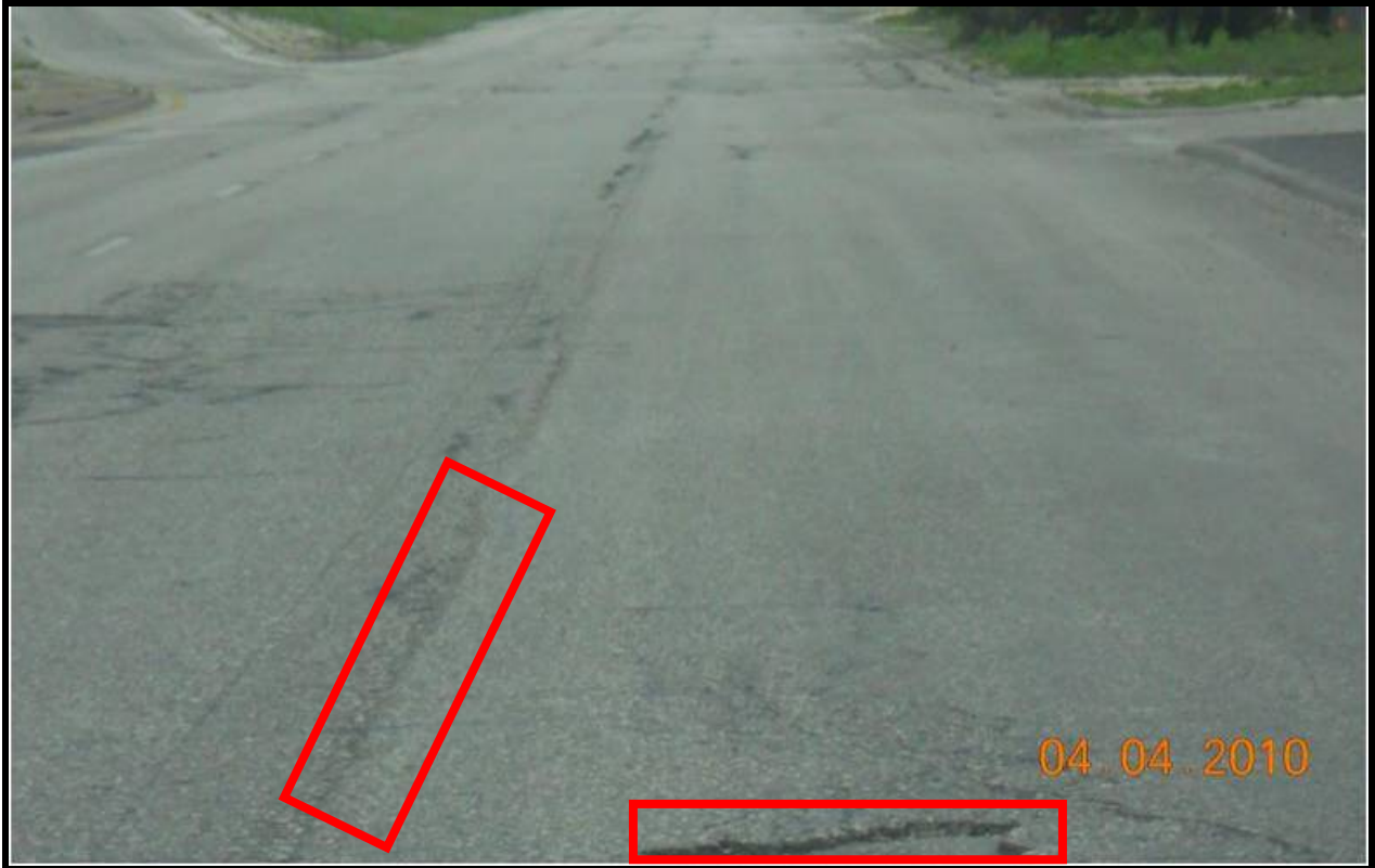
Category 4: IH 410 SB+NB FR from FM 78 to Rittiman (potholes and long. and trans. cracking)
