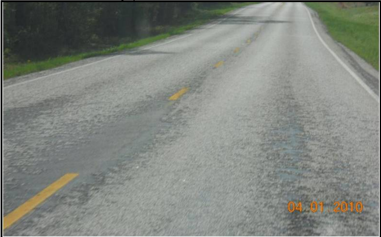
Category 2: FM 322 from SL 256 to SH 294 (shallow rutting and raveling)
