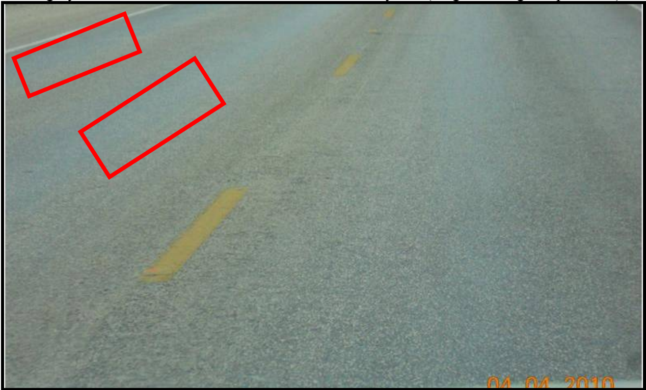
Category 2: FM 1535 (wheel path rutting)
