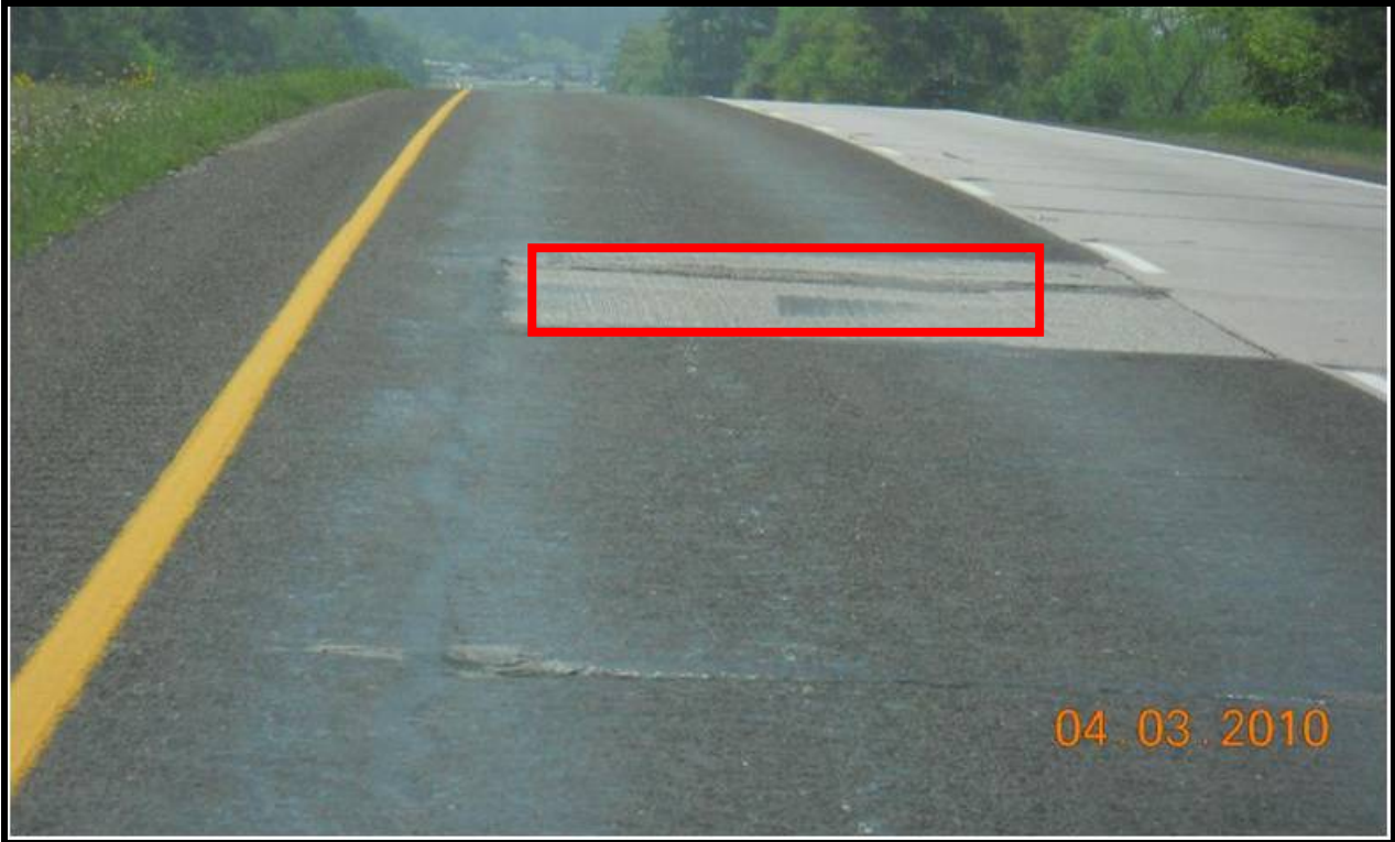
Category 4: Southbound US 59 (Livingston city limits) (reflective cracking)
