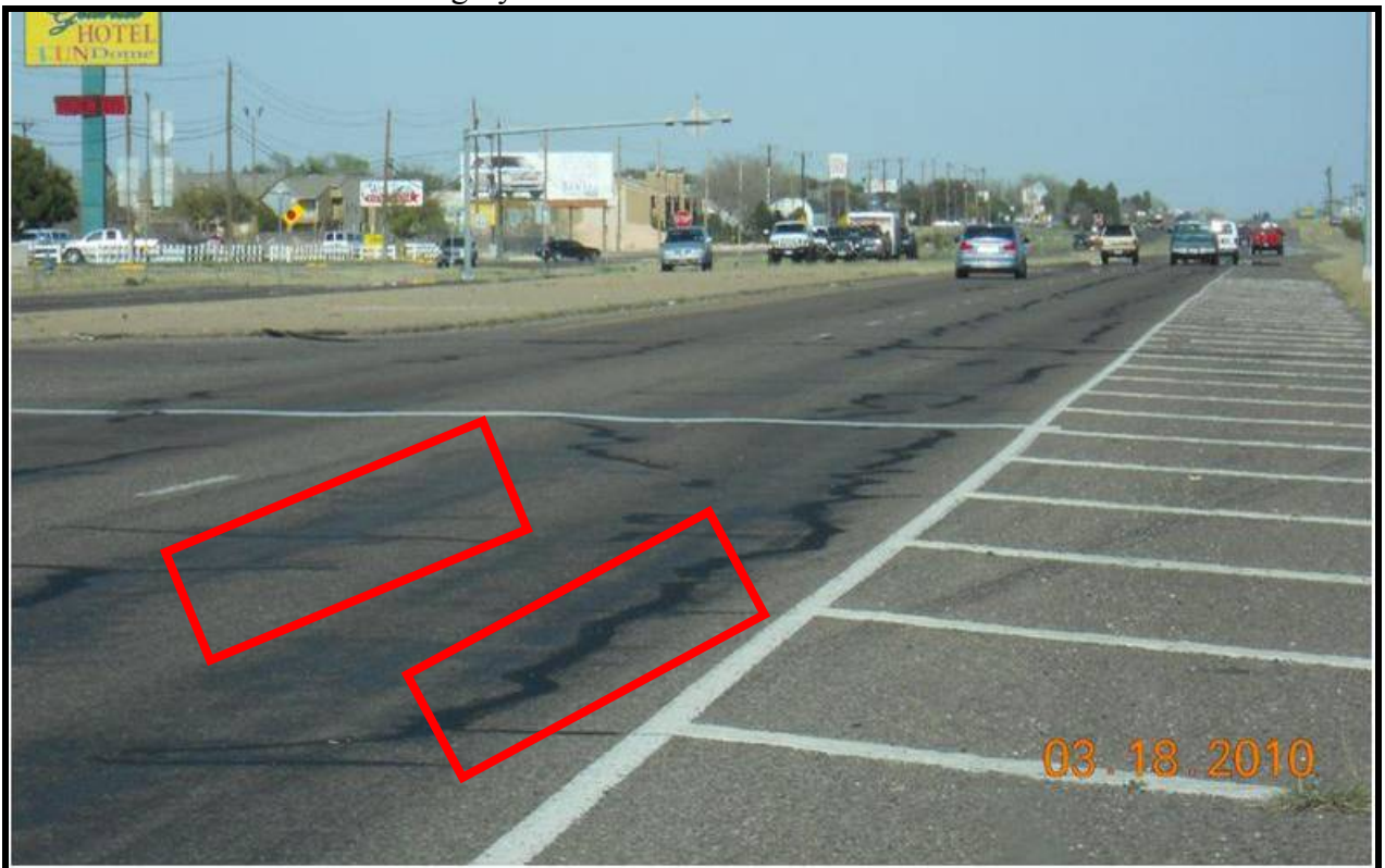
Category 5: BI 20 from SL 250 to SL 338 (wheel path rutting)
