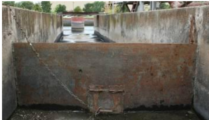
Figure 3.12. Sharp Crested Weir.
