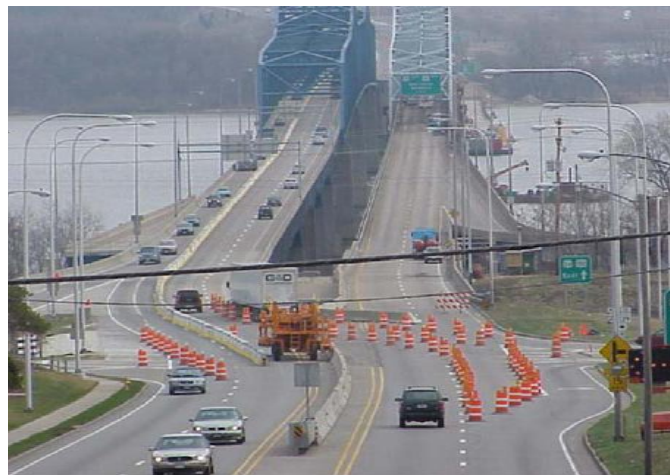
Figure 1.1. Temporary Concrete Traffic Barrier in Construction Zone.
