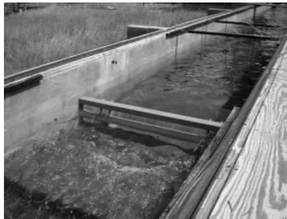
Figure 2.10. Rail in the Rectangular Channel.
