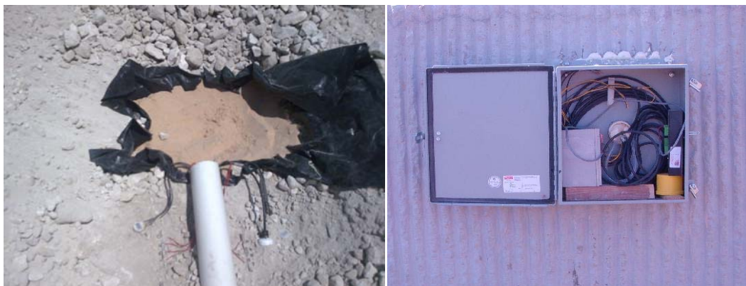
Figure 7.3 – Sensor Placement and Metallic Enclosure from Completed Site.
