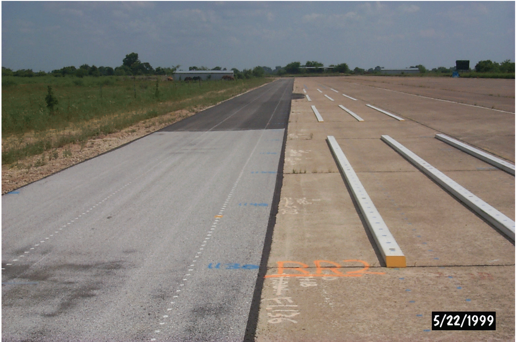
Figure A9. Start of Section RR2 at Ride/Rut Facility (Rut Calibration Bumps at Right of Photo).
