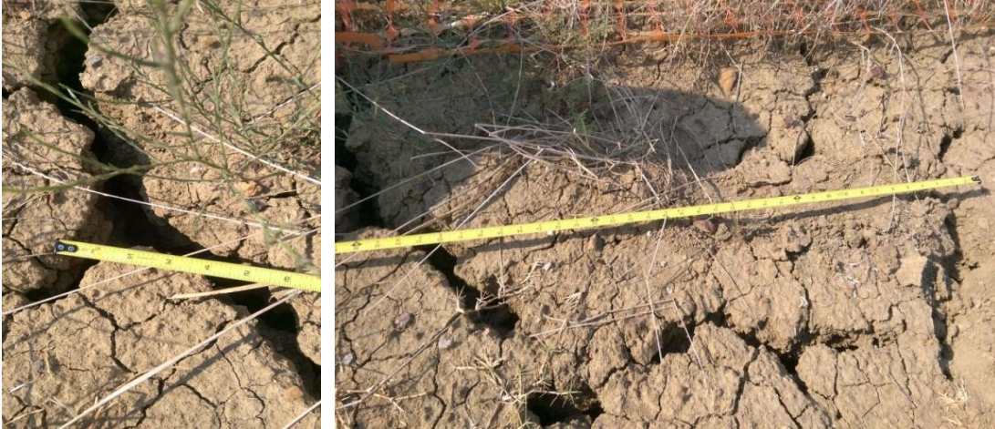
Figure 13: Cracks observed at test section 3 (control section)
