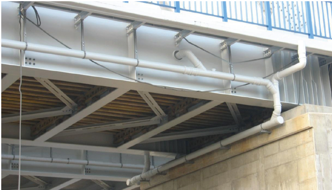
Figure 2.10 Pipes along the bridge deck with the same color as the steel beams (Vlčeka, 2012)
