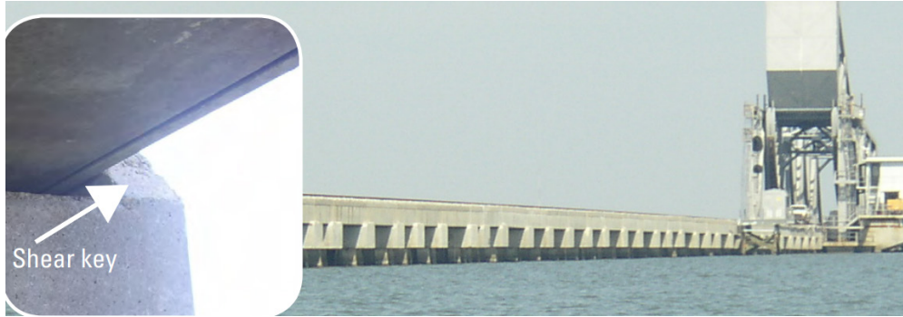
Figure 2.10 Railway bridge adjacent to the I-10 twin span bridge between New Orleans and Slidell (Chen et al., 2005)
