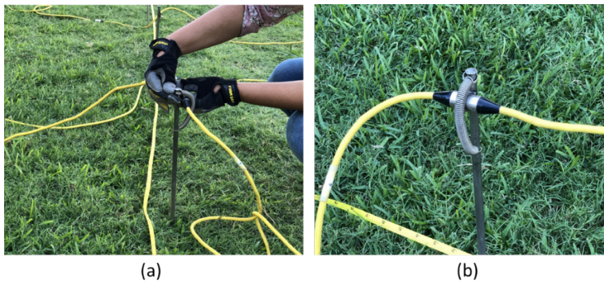
Figure 3.22 (a) attachment of a cable to an electrode using a stainless-steel spring and (b) the appropriate connection of a cable take-out to an electrode
