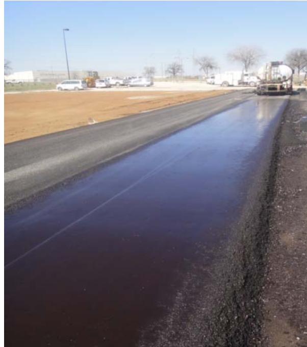
Figure 5.2. Tack Coat Application on Section H prior to Placement of the Final Lift (CSS—1H @ 0.05 gal/sq yd).
