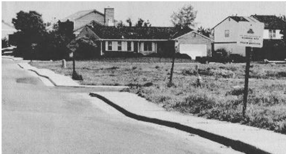
Figure 2.3 Pavement overlying expansive soils and subjected to distress due to shrink-swell movements (Source: www.surevoid.com )
