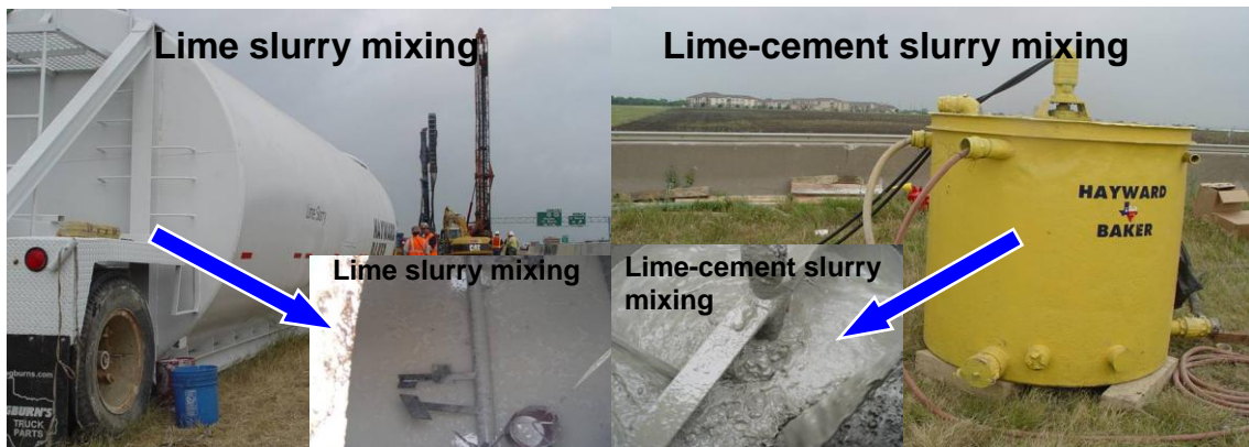
Figure 5.14 Mixing tanks used for the preparation of lime-cement slurry
