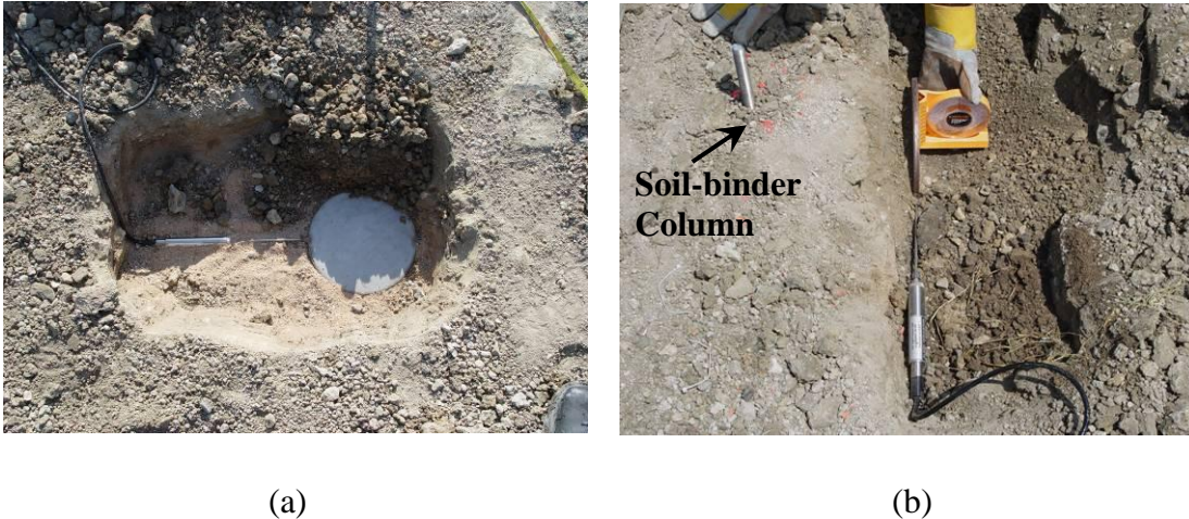
Figure 5.32 Schematic of pressure cell installation (a) Horizontal orientation and (b) Vertical orientation
