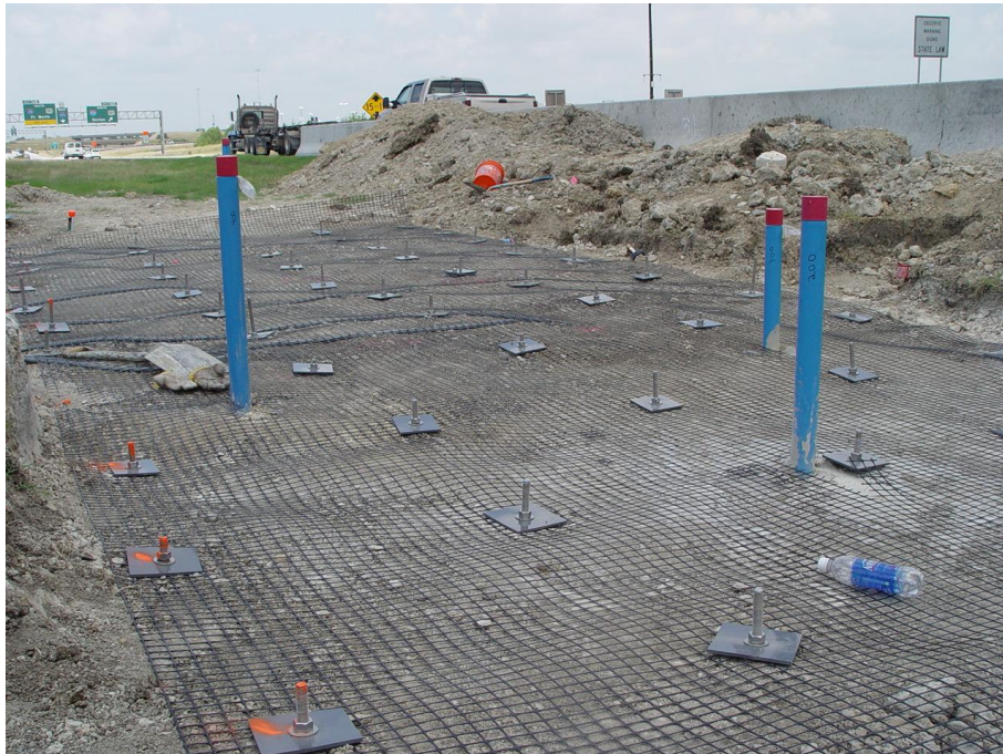
Figure 5.19 Test section after fastening geogrid to DSM columns using anchor rod and plate-bolt system.
